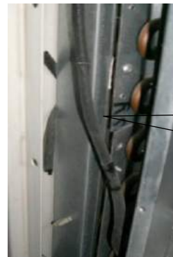
After being reconnected, the system becomes normal
