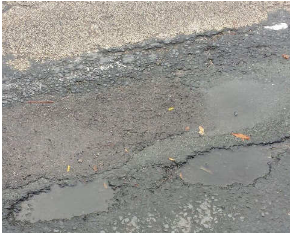
Figure 6 - Highway Defect on Chester Street
