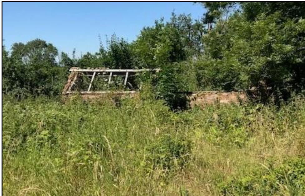
Photograph 13 showing the dilapidated shippon
