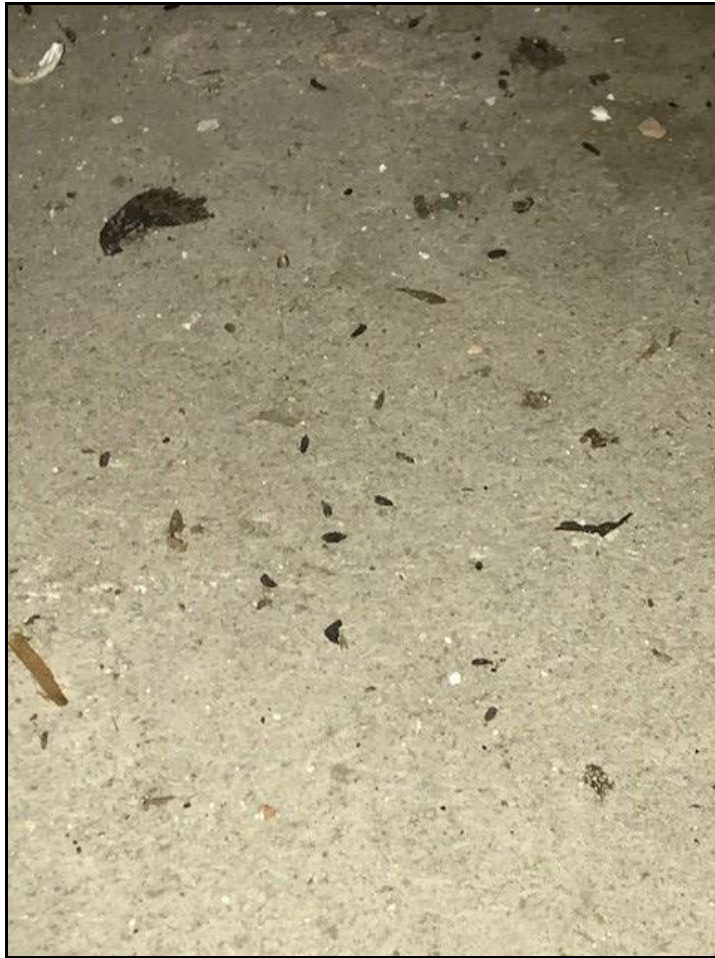
Photograph 8 showing bat droppings and feeding remains
