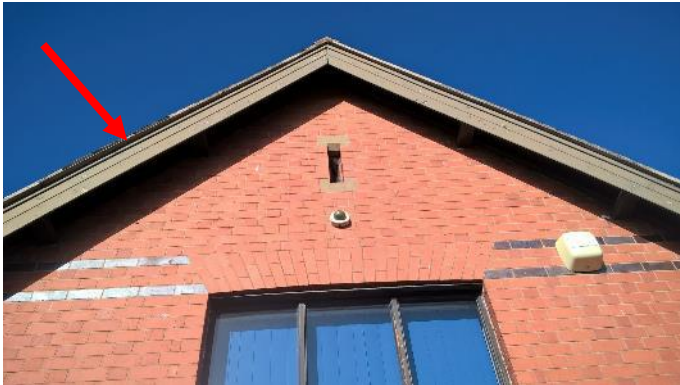
PICTURE 9. THE SOUTHERN GABLE. THE ARROW INDICATES GAPS WHERE MORTAR HAS FALLEN FROM UNDER SLATES.
