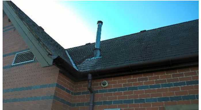
PICTURE 10. GAPS AROUND CHIMNEY FLASHING.
