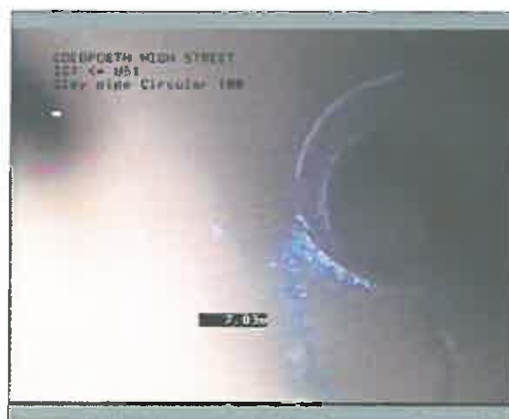
Photo: 3_1_8_23022017_144817_A.jpg 7.03m, Broken pipe at joint, from 6 to 8 o'clock
