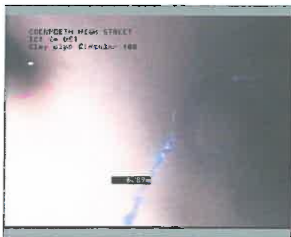
Photo: 3_1_4_23022017_144735_A.jpg 6.89m, Fracture, longitudinal at joint, at 9 o'clock
