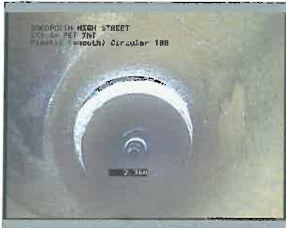
Photo: 1_1_3_23022017_135220_A.JPG 2.36m, Joint displaced, medium
