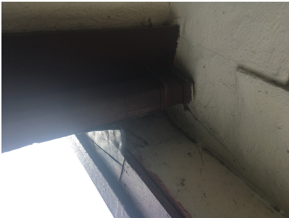
Plate 8: Gap in flashing where roofs adjoin
