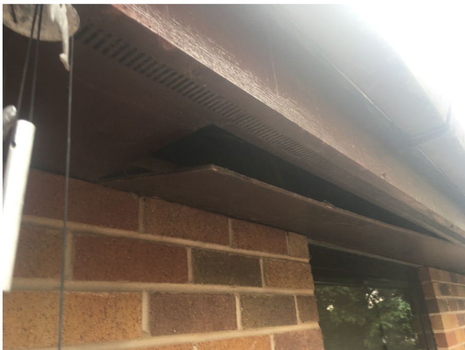
Plate 4: Example of damaged soffit
