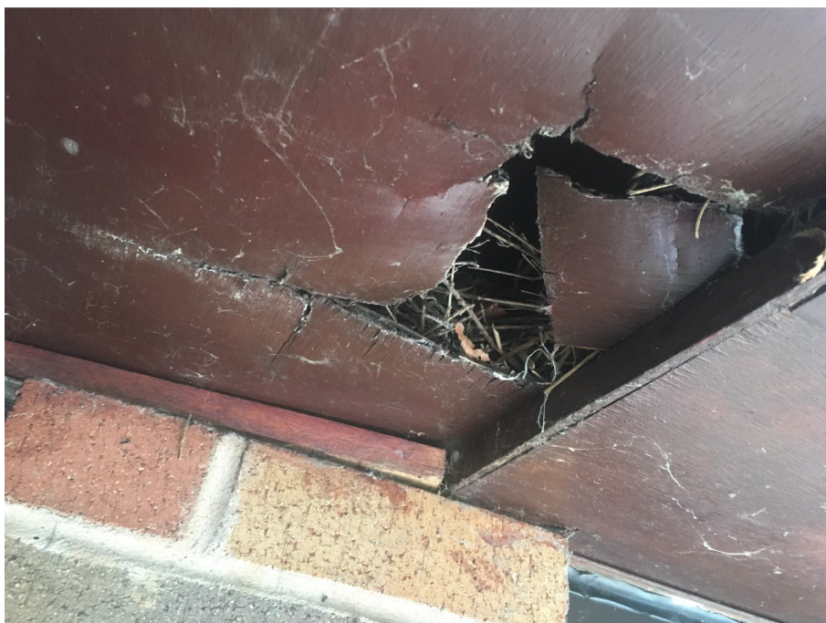
Plate 5: Damaged soffit with bird nesting material within soffit box
