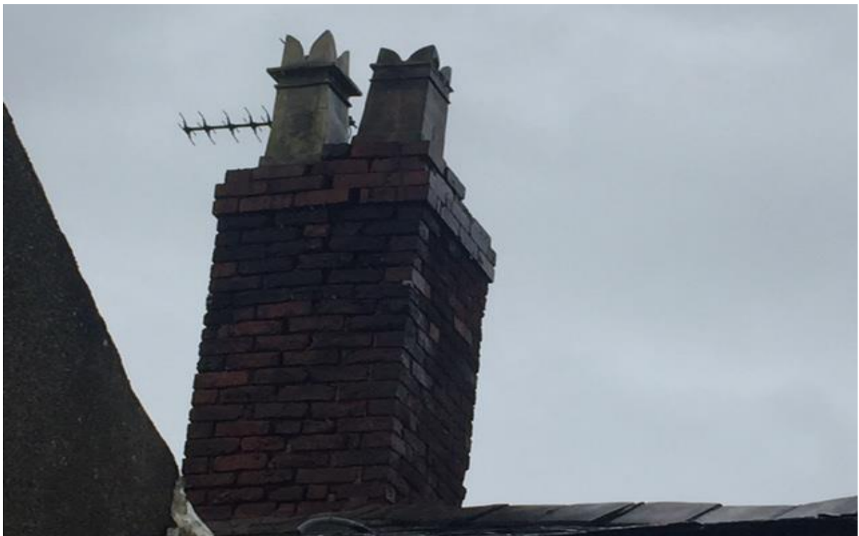
Central chimney with large vertical crack and unstable brick work.
