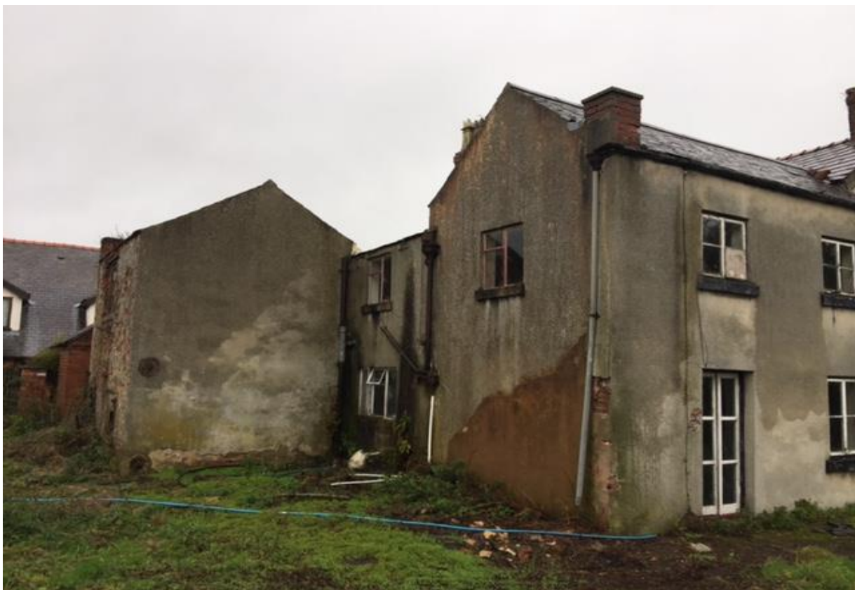
Elevation showing the older section of the property – note very poor brick work to the far elevation that will require partial re-build.
