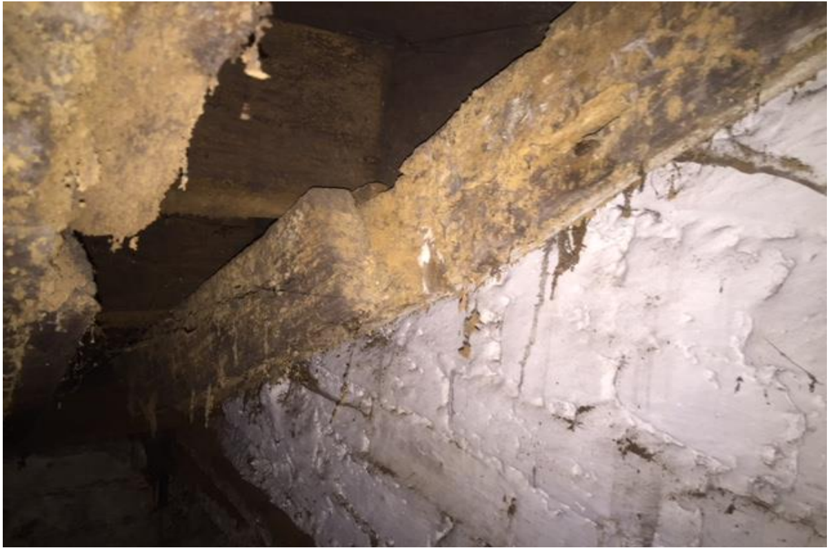
Failed and rotten timbers supporting stairs.
