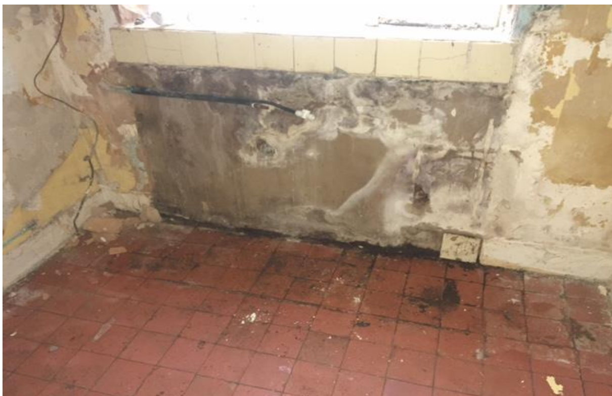
Damp walls and floor to rear elevation rooms due to high external levels and lack of membrane.
