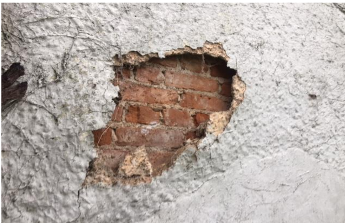
Some of the walls under the render appeared in fair condition, particularly to the north east and south-east elevations.
