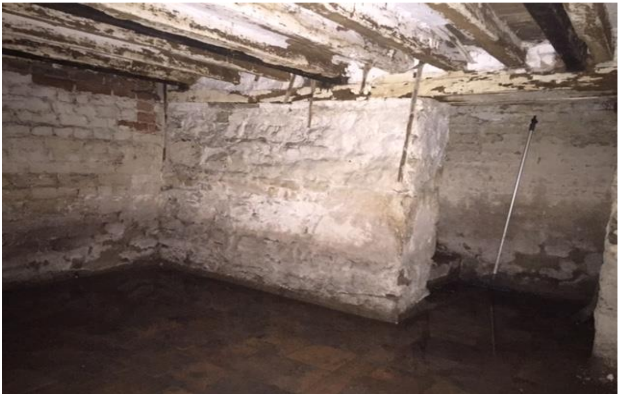
Damp environment within basement
