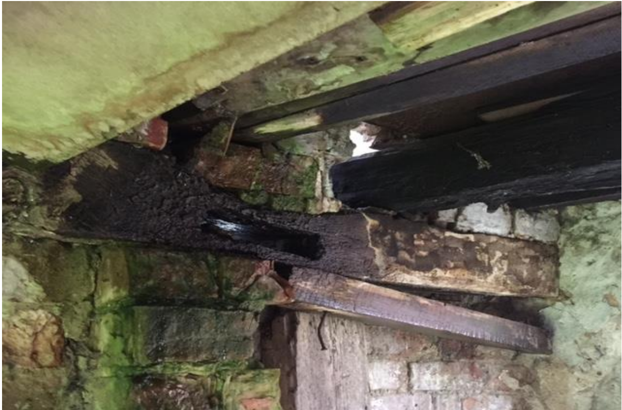
Some of the internal timber and roof elements require complete replacement.
