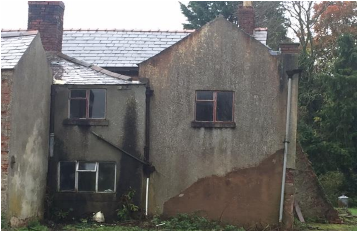
Rear elevation – note, external levels above internal floor and leaning wall with buttress.
