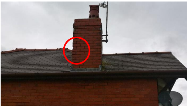
Plate 4.11: B2 – Missing Mortar on Chimney
