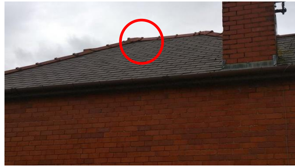
Plate 4.10: B2 – Gaps Under Ridge Tiles
