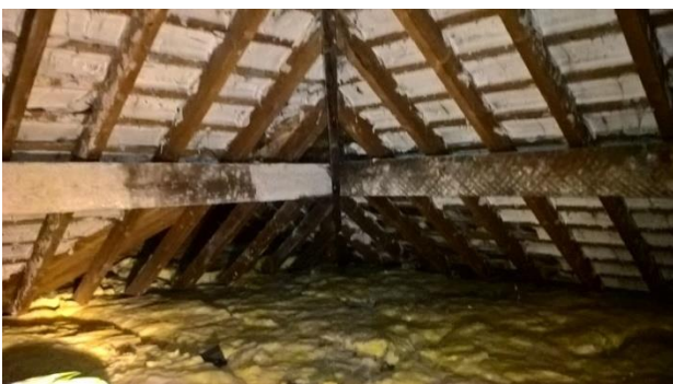
Plate 4.19: B2 – Internal Roof Space, Showing Plaster on Tiles and Insulation on Floor
