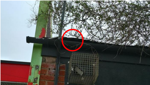
Plate 4.3: B1 – North-Western Elevation Showing Gaps Under Corrugations
