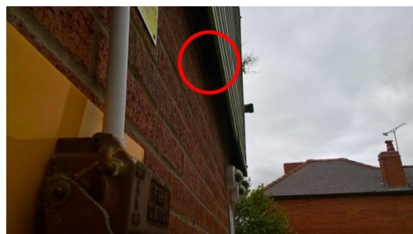
Plate 4.2: B1 – North-Eastern Elevation, Gap Between Wall and Metal Frontage
