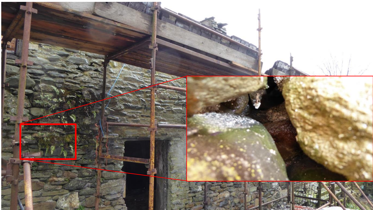
Figure 4.3. Gap shown in brickwork
