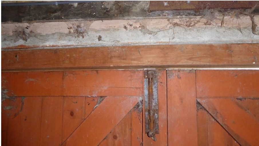
Figure 4.6. Crack above doorway large enough for bats
