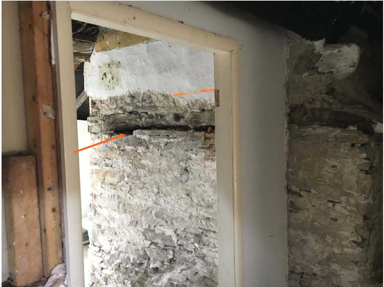
Photo B: Bathroom chimney lintel crevice.
