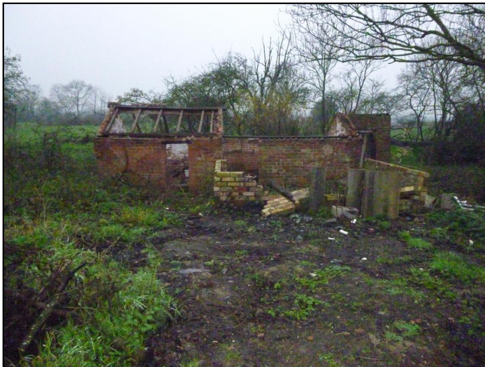
Photograph 9 showing the dilapidated shippon
