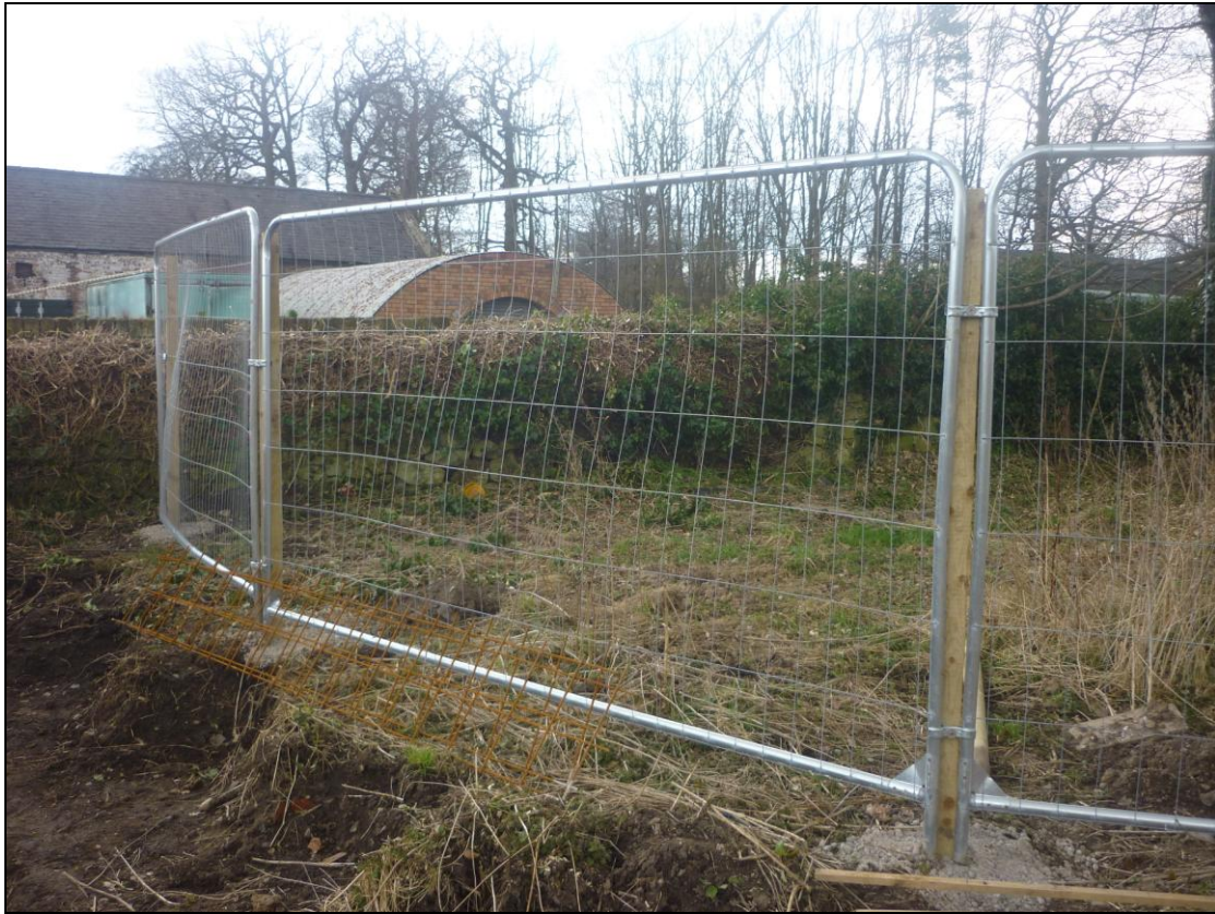
Photo 3 - Fencing around T1
