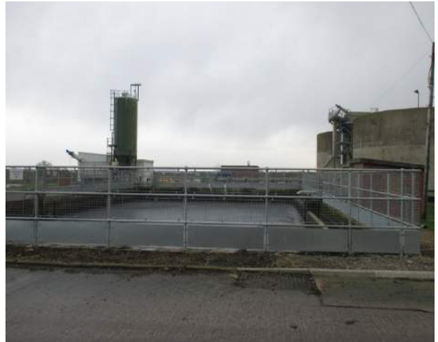
Photo E.40: Post digestion tank
