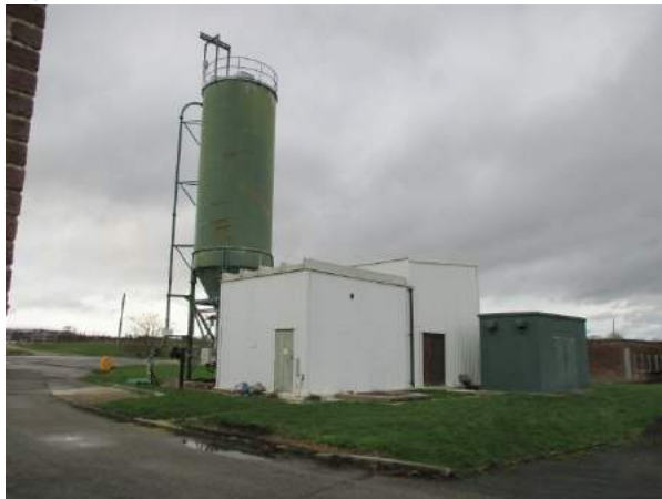
Photo E.5: Lime silo with the lime plant building adjacent
