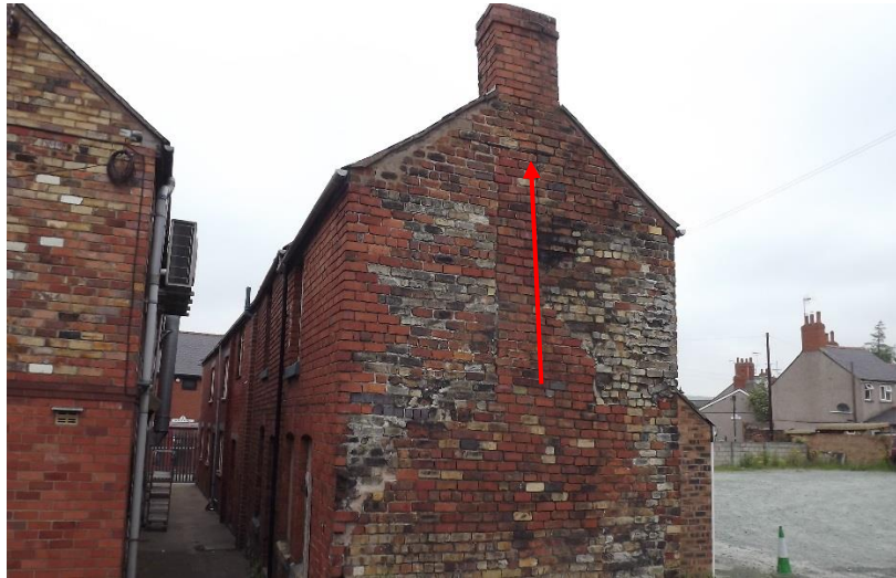
Image 3.2 Eastern aspect of the building showing the raised bricks depicted by the red arrow.
