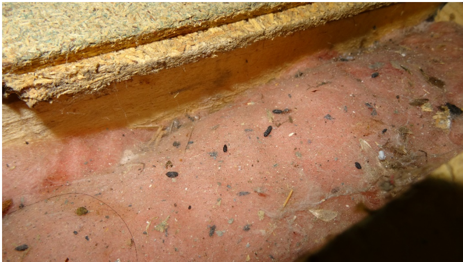
Figure 7. The droppings found in the loft space, all were rodent droppings
