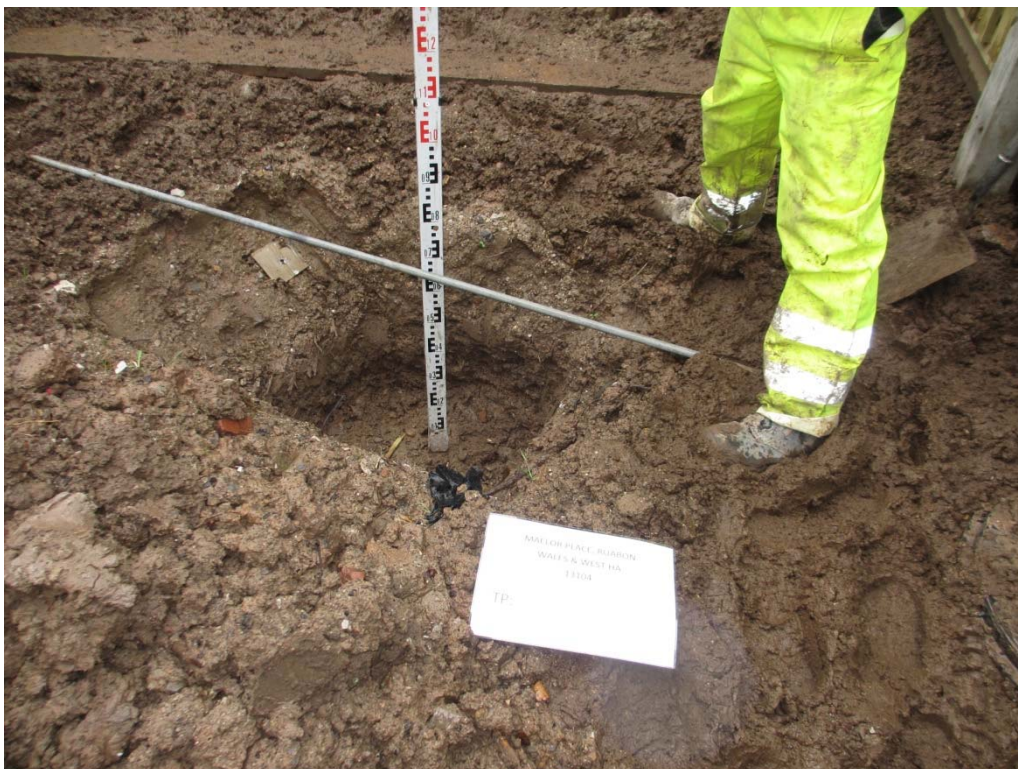
Photo 6 – Plot showing capping thickness >0.60\text{m} at Plot 11
