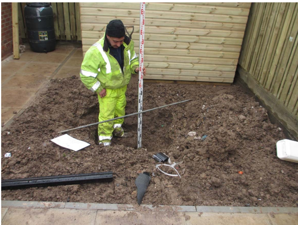
Photo 10 – Plot showing capping thickness >0.60\text{m} at Plot 18
