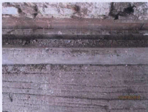
Figure 10: floor and wall area in Section 1. Bat droppings were found here in 2008 and it was concluded that a feeding roost may be present.
