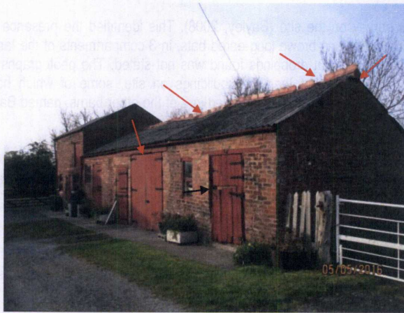
Figure 11: potential access points for bats
