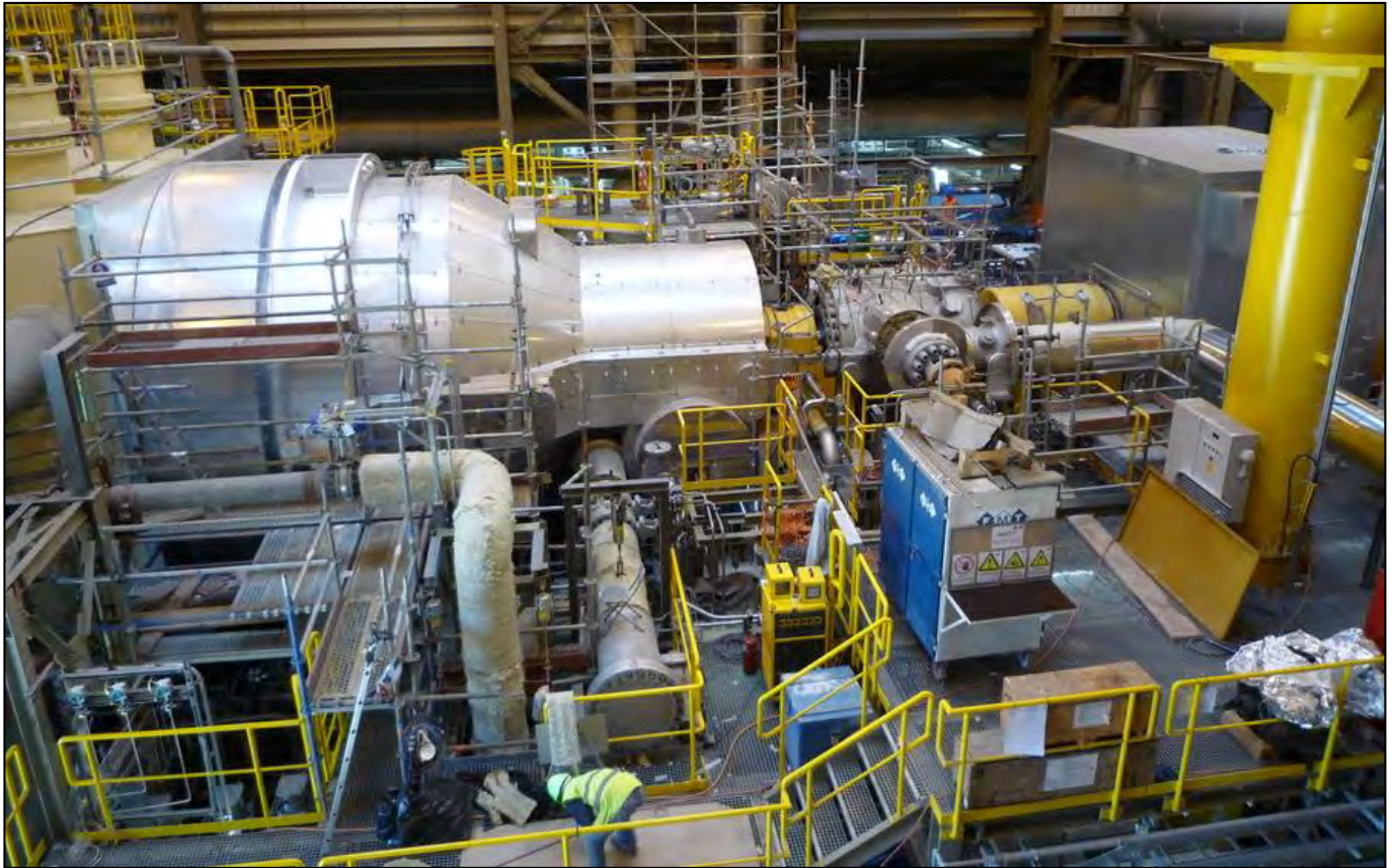
Figure DAS24: Interior of a typical CCGT power station turbine hall. For illustrative purposes only.
