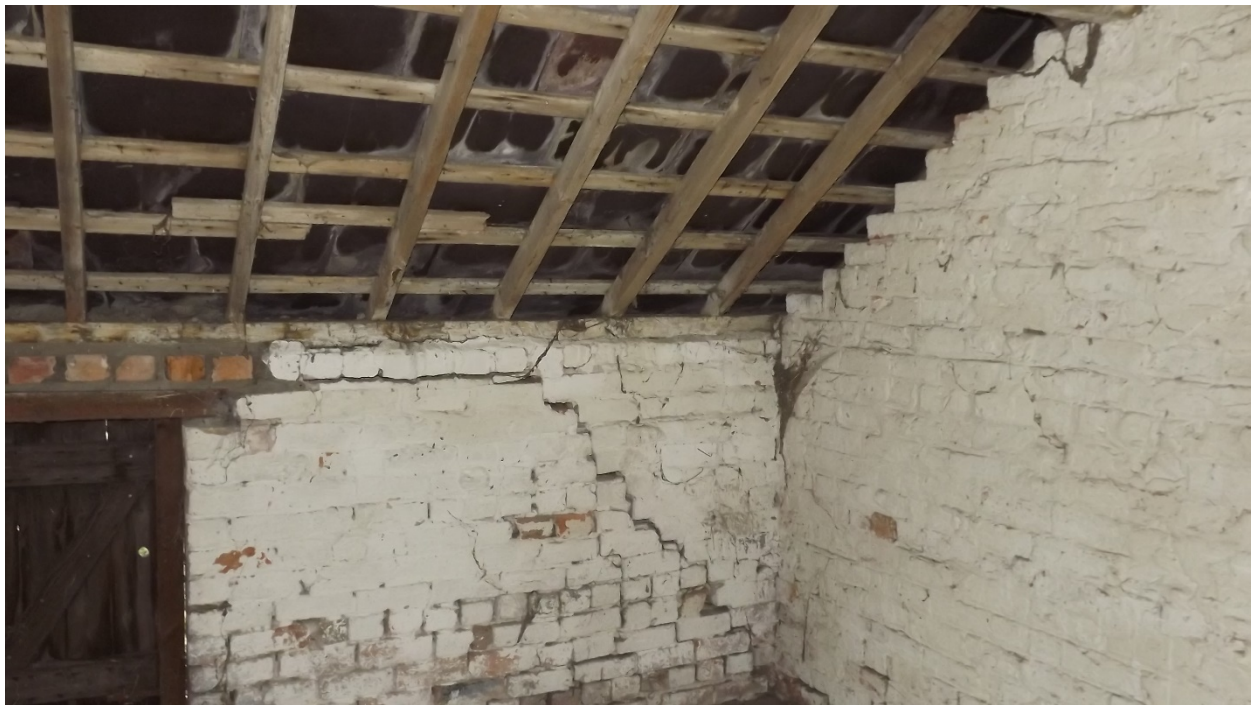
Figure 5. Showing the upper floor of the north building, showing the unlined timber roof and general damage to the brickwork
