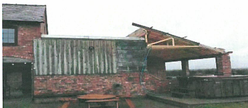
Section to the south on which a roof covering is not present
