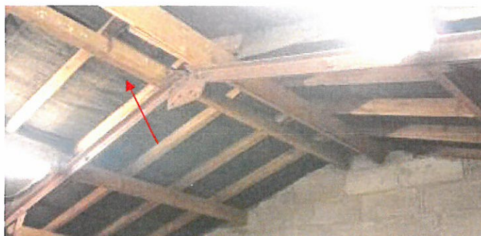
Bird droppings on internal beams
