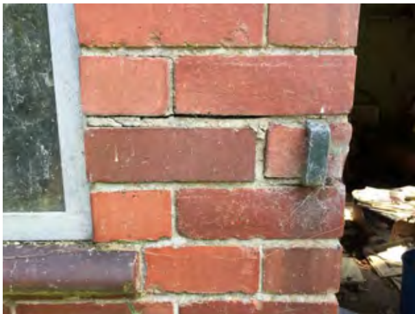
Cracked brickwork due to corrosion of embedded steelwork.
