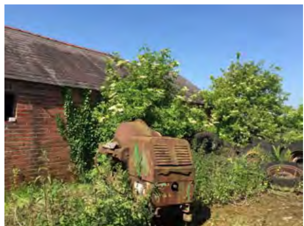
Vegetation masking the rear elevation.
