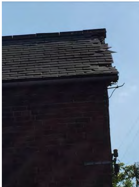
Condition of verge considered to be poor.
