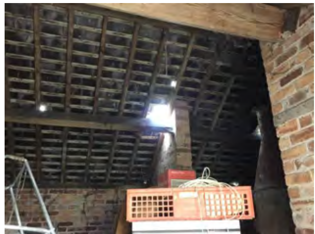
Holes through roof over rooms 1 and 2.
