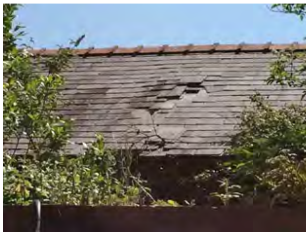
Slipped tiles and hole through roof.
