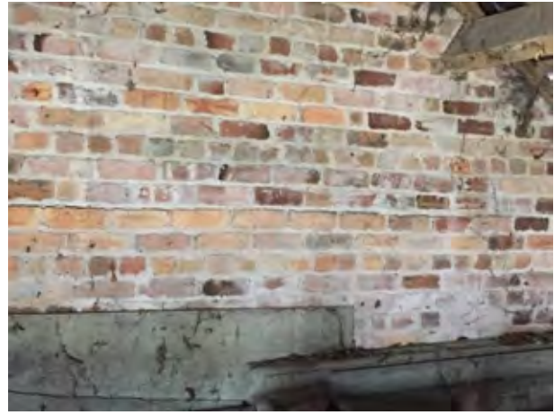
Cracking continues across gable wall.
