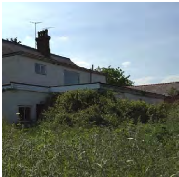
Rear elevation of rear extensions. Vegetation covering elevations.
