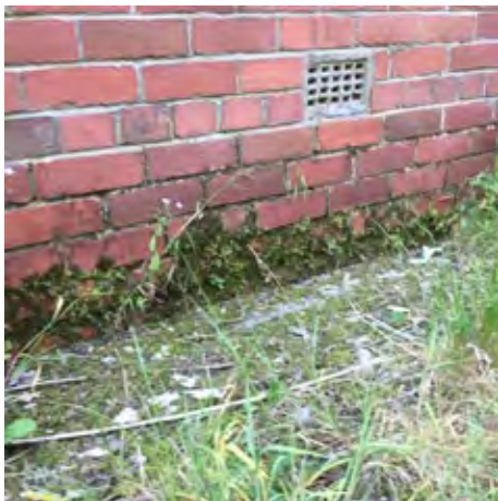
Moss growth indicating possible damp.
