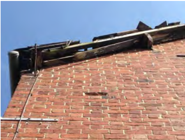
Timbers and fascia boards to eaves are rotten and the slates are missing or damaged.
