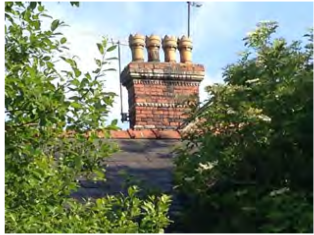
Water staining to main chimney stack.
