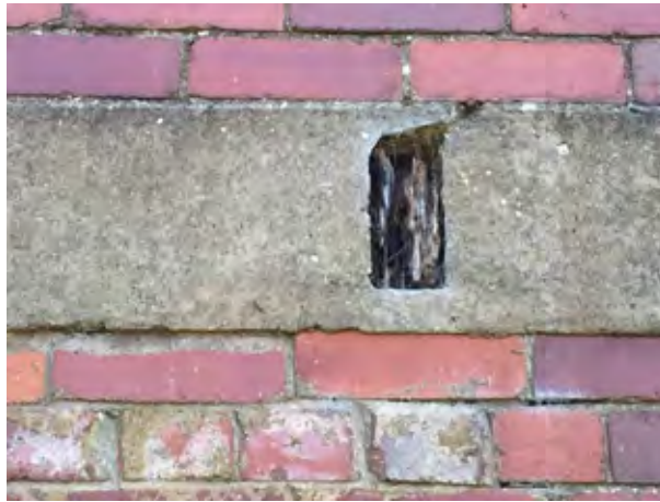
Rotten timbers within concrete ring beam.
