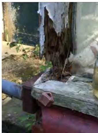
Rotting timber fascia to side extension.
