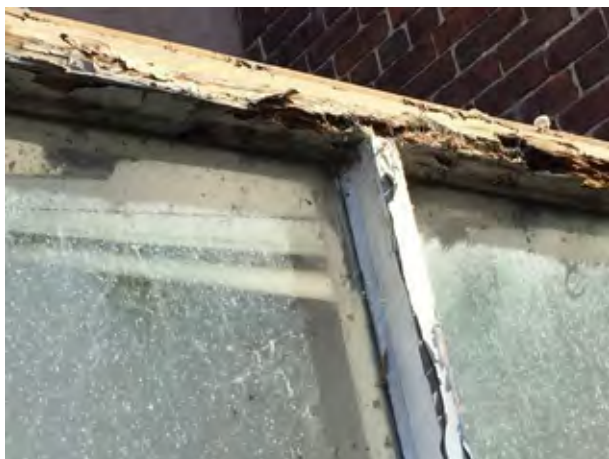
Rotting timbers to rear porch structure.
