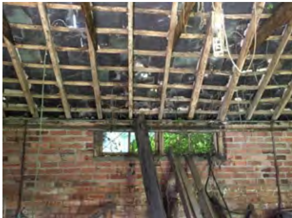
Deflecting roof timbers.
