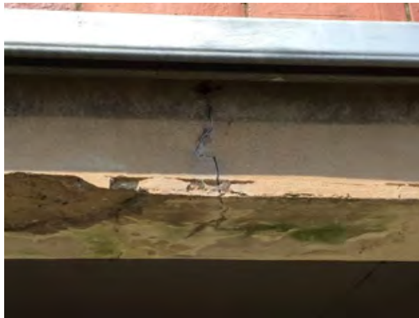
Concrete lintel cracked.
