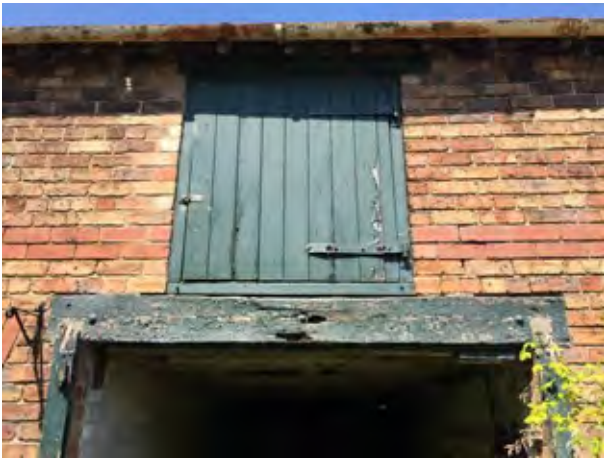
Deflecting and weathered timber lintel.
