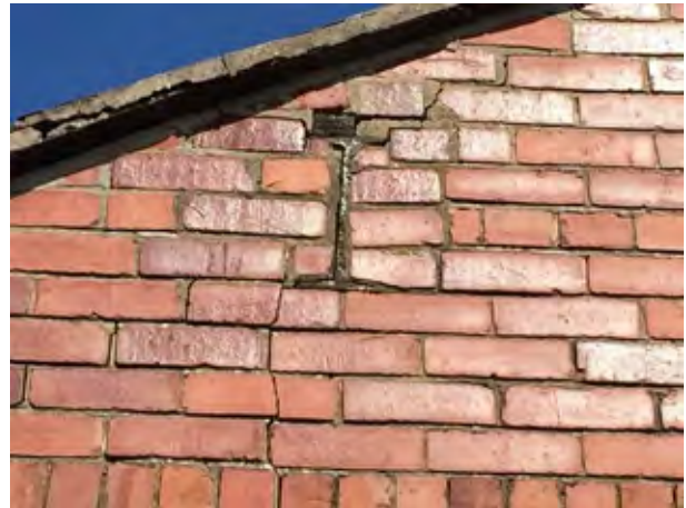
Corroding steel purlins have caused cracks to form in the brickwork.
