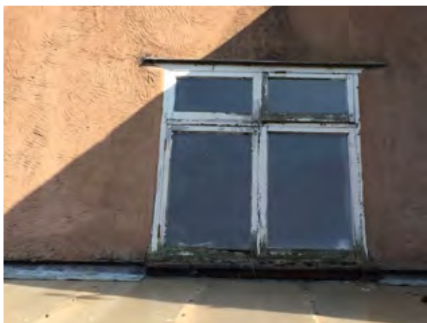
First floor timber window frame rotting.
