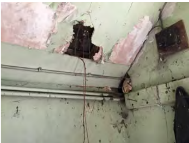
Holes through roof within Room 1.
