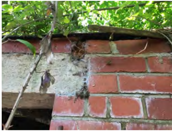
Missing eaves structure.
