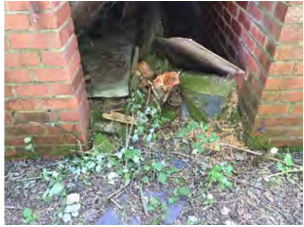
Tree growing within the doorway.
