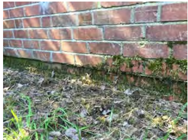
Moss growth at low level indicating damp ingress. The brick elevation has moved outwards at low level.
