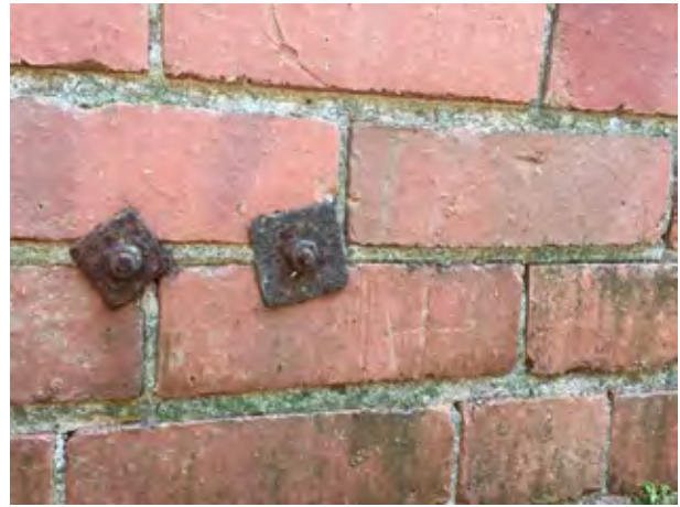
Corroded embedded steelwork has caused a horizontal crack to form.
