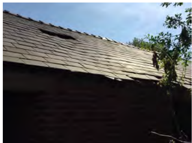
Holes through roof, missing and slipped slates and missing rain water goods.
