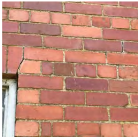
Cracking to right hand, rear corner masonry.
