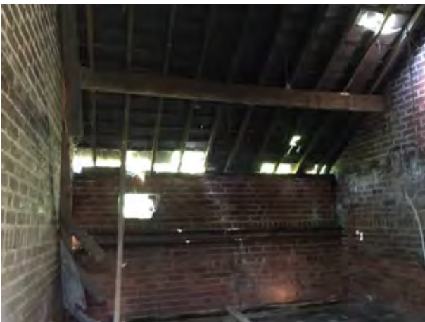
Holes through roof and rear wall.
