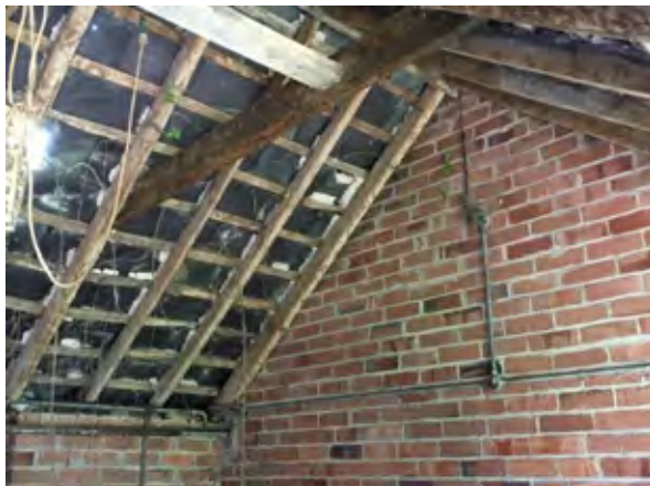
Holes through roof structure.
