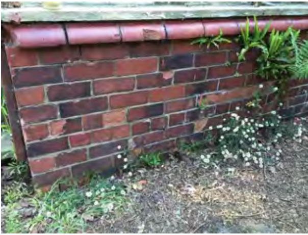
Spalling bricks to rear porch structure.
