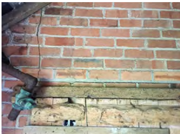
Cracking over lintel in cross wall.
