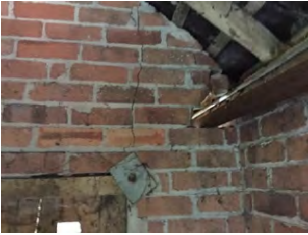
Cracking over lintel in cross wall.
