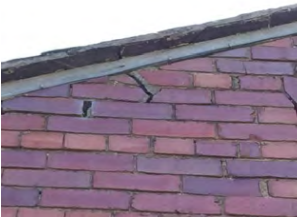
Cracking to brickwork where steel purlins are built into the masonry.
