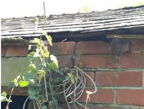
Slates are missing; vegetation is growing within the masonry and cracked and loose brickwork.
