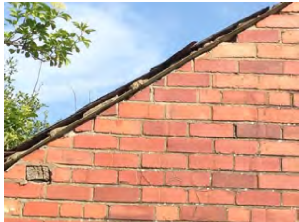
Mortar dislodged from verges.
