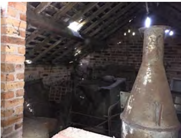
Holes through roof over rooms 2 and 3.
