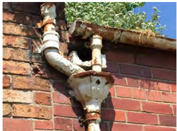
Holes through elevation.
