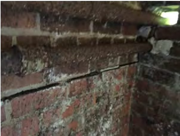
Horizontal cracking to right hand side gable wall.
