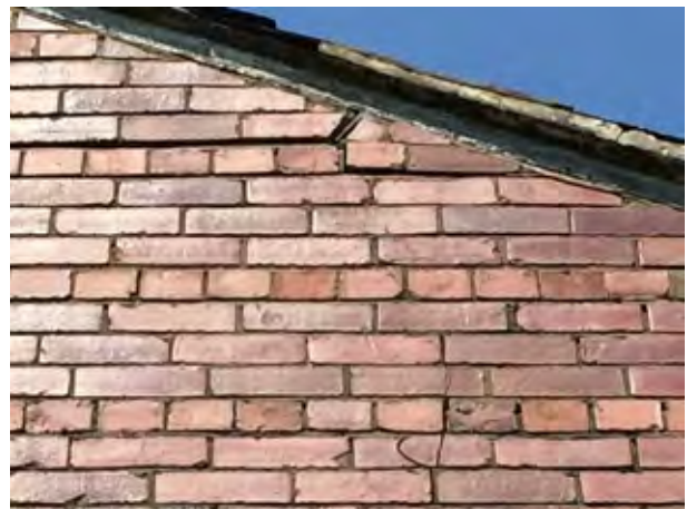
Cracking and lifting brickwork where purlin end built into elevation.
