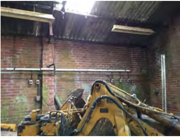
Water staining on rear wall.
