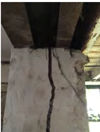
Cracking to bearing below steelwork in Room 4.
