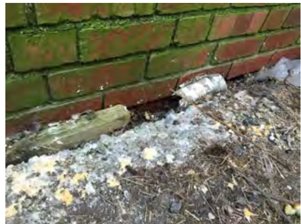
Movement of brickwork outwards at low level.
