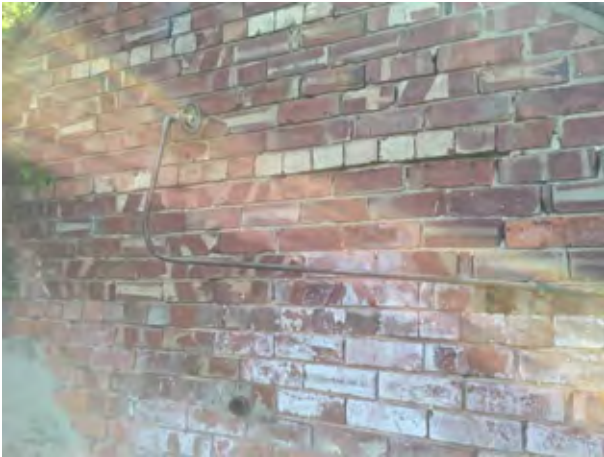
Mortar weathered to left hand side elevation.
