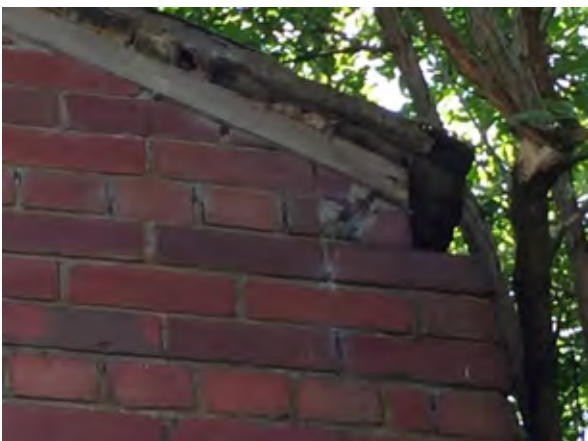
Damage to eaves and verges.
