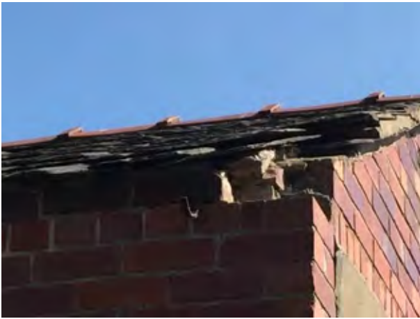
Missing rain water goods, damaged eaves and missing slates.
