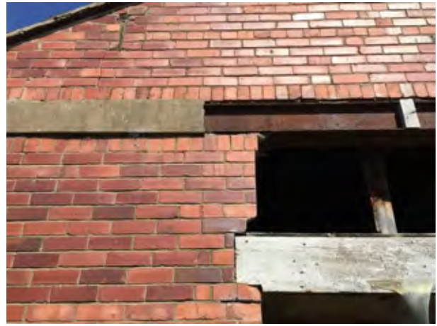
Concrete dislodged from corroding steelwork.
