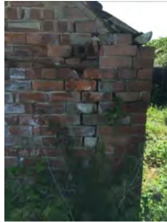
Movement of piers / buttress and damage to brickwork due to pipe penetration.
