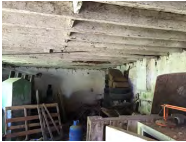
Over deflecting floor joists over Room 4.
