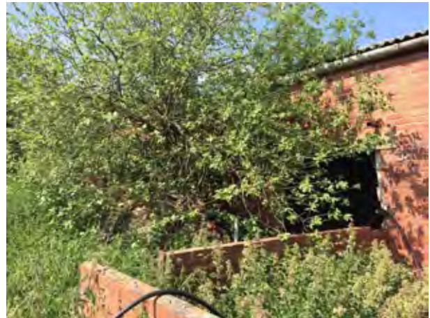
Trees built close up to the rear elevation.
