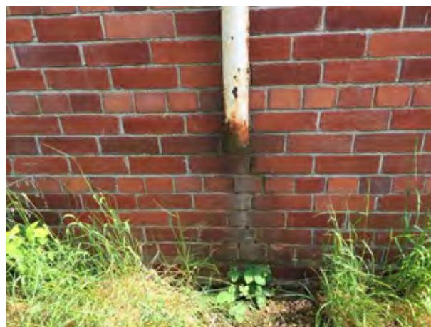
Missing rain water goods.
