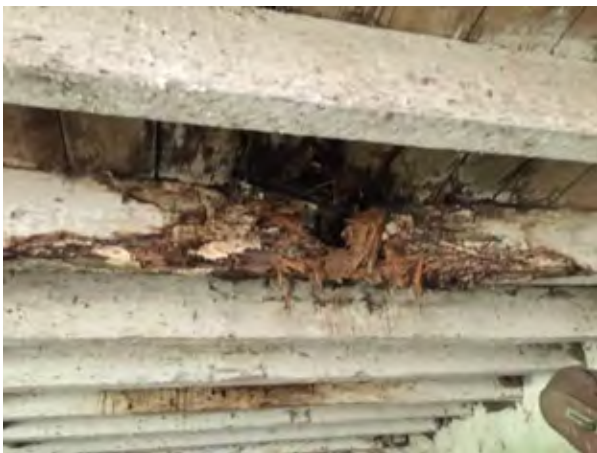
Hole through floor in Room 4.
