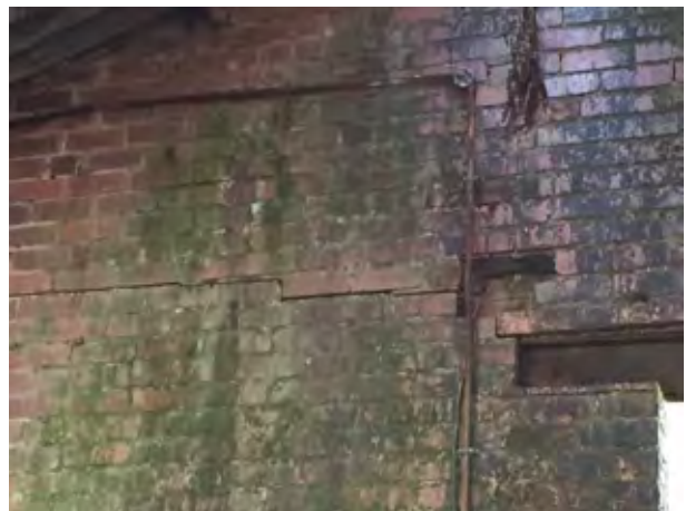
Cracking to right hand side wall.
