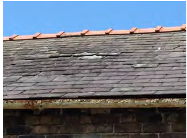
Holes through roof. Slipped tiles.
