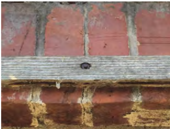
A fixing through the timber has caused the standing soldier lintel brickwork to crack.
