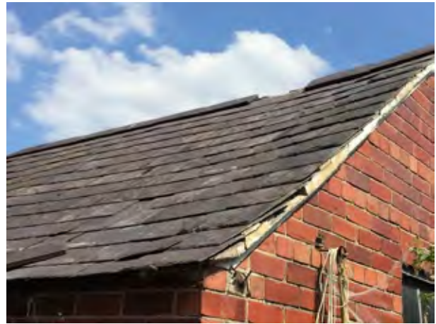
Slipped slated and ridge tiles.
