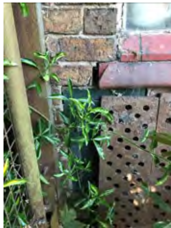
Cracking below window to Room 1.
