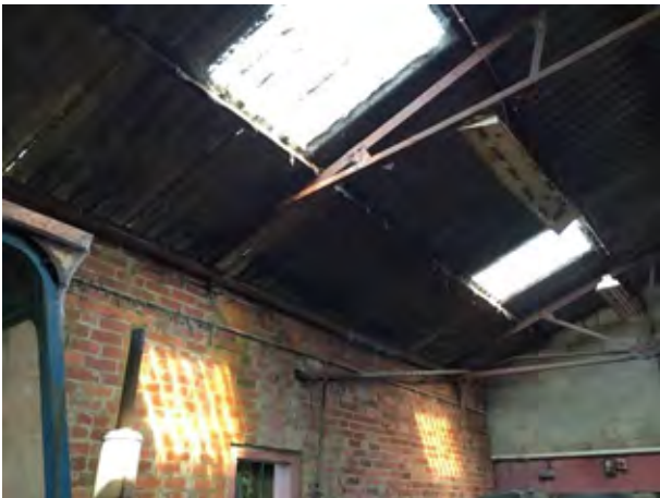
Bottom chord missing from steel truss.
