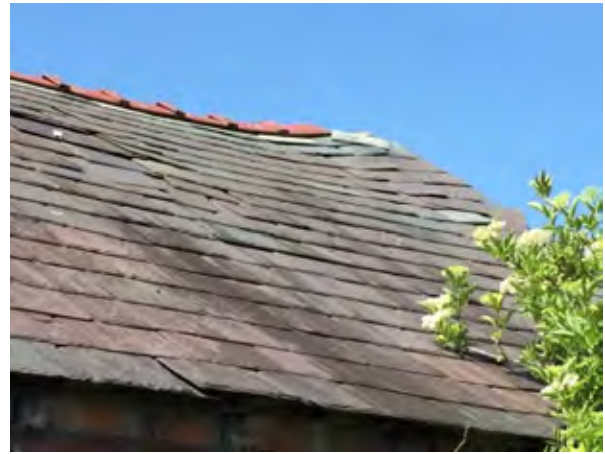
Undulating roof slopes noted.
