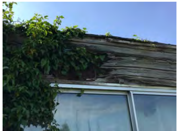
Rotting timber fascia to side extension.
