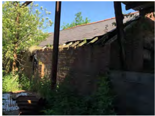
Holes through roof and missing slates at eaves level.
