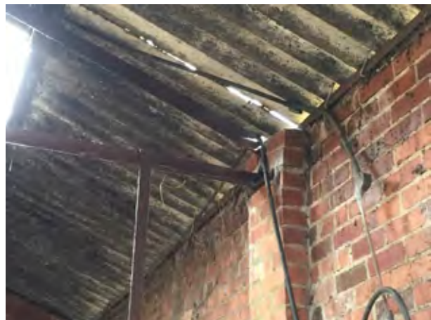
Trusses supported by brick piers. Brickwork lifted.
