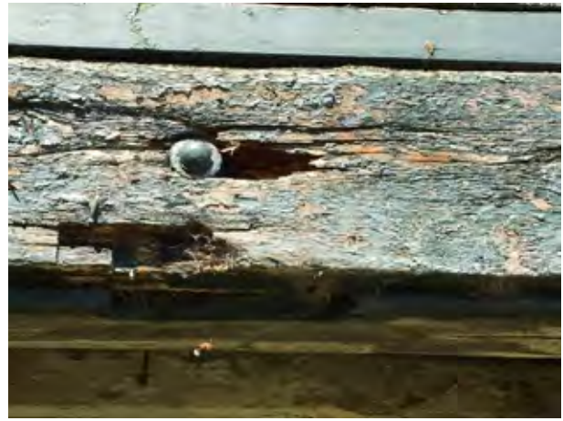
Weathered timber lintel.
