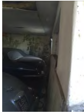
Rear wall leaning outwards.
