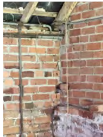
Crack formed between cross wall and front elevation wall.
