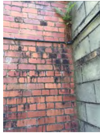
Water staining to front elevation brickwork.
