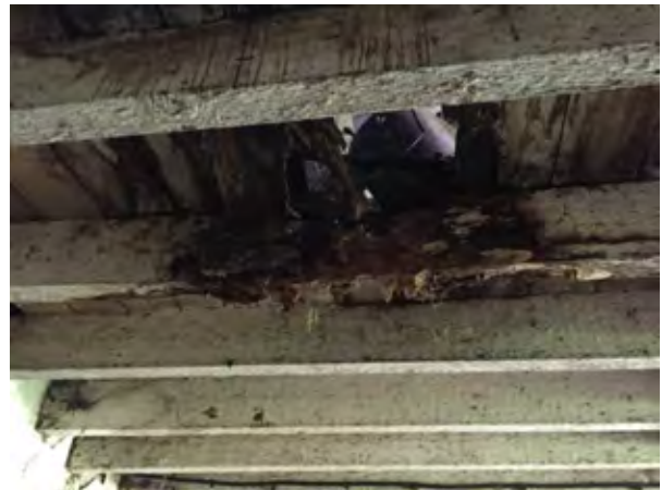
Hole through floor in Room 4.
