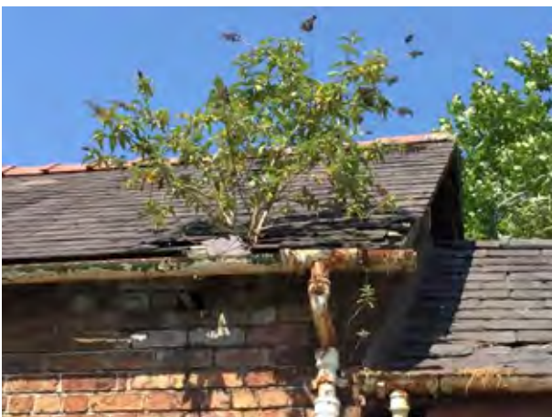
Vegetation growing through the structure.
