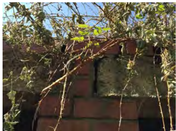
Gaps adjacent to lintels. Vegetation growing through the structure.
