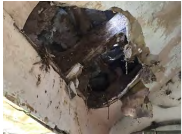
Rotten rafter ends visible.
