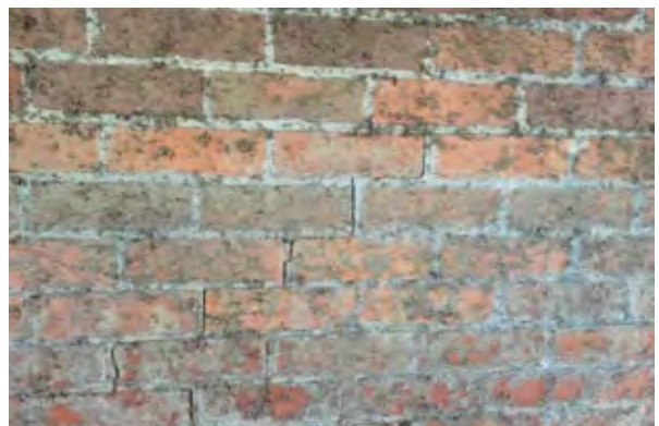
Cracking to cross wall.
