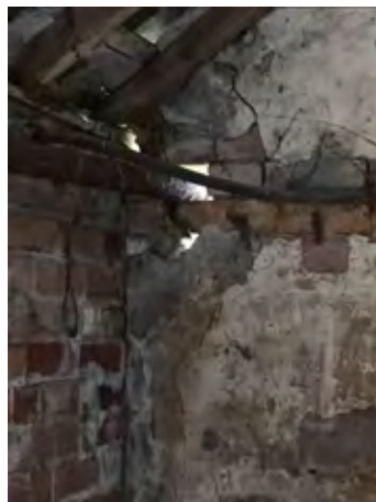
Hole through left hand side gable wall.
