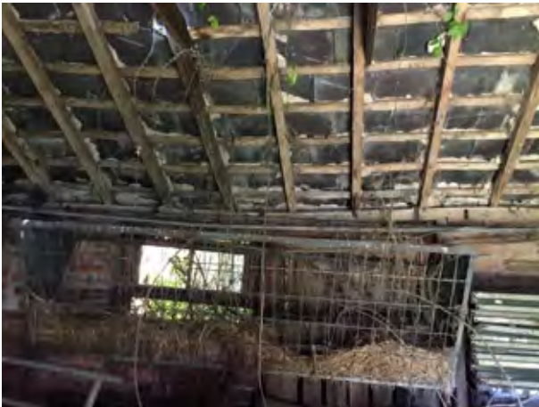
Over-deflection of rafters and wall plate which also acts as a lintel.
