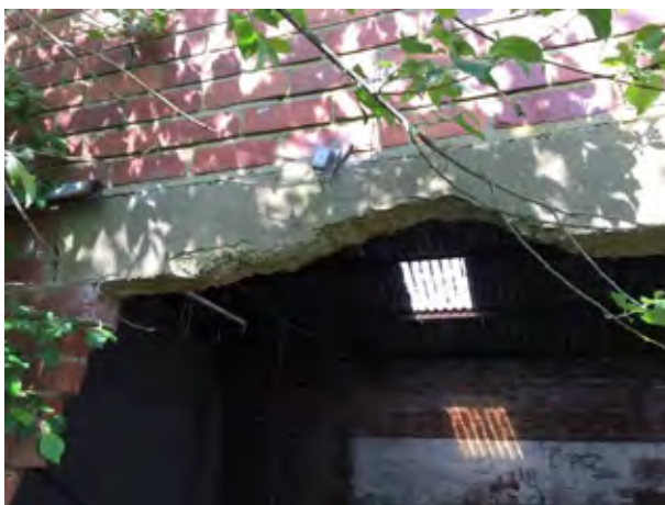
Damage to lintel over poorly widened opening through rear wall.
