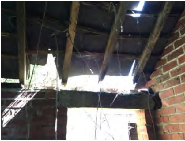
Missing structure at eaves.
