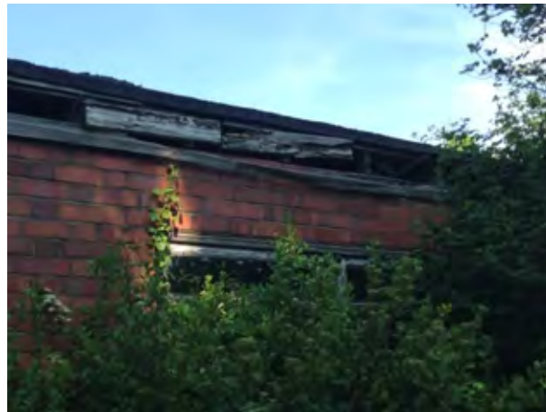
Fascia boards dislodging, exposing flat roof joist ends.
