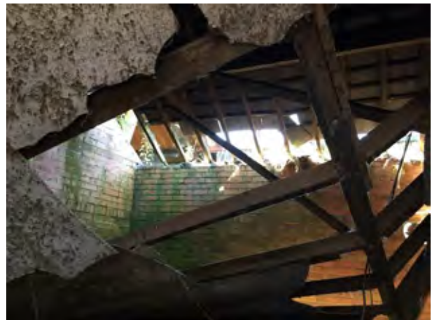
Ceilings collapsing and holed noted through the roof structure.
