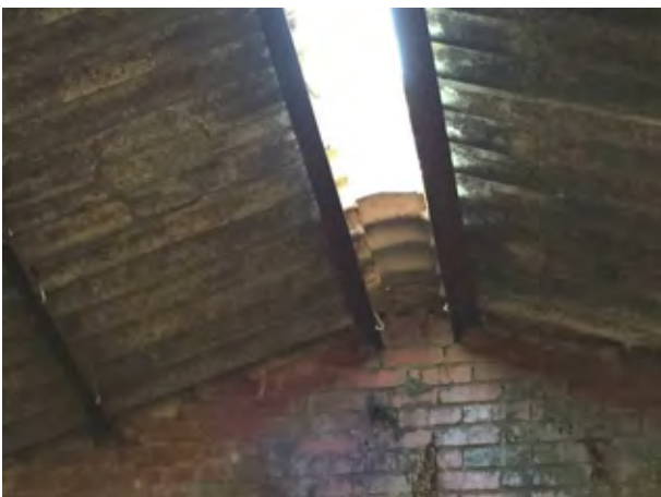
Roof sheeting missing.
