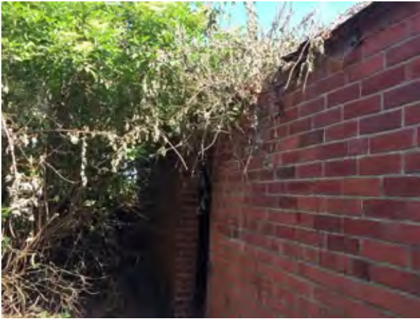
Vegetation obscuring the elevations and growing through the masonry.
