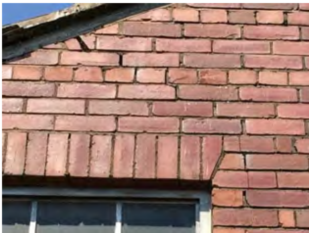
Cracking to elevation where purlin end built into the external elevation.
