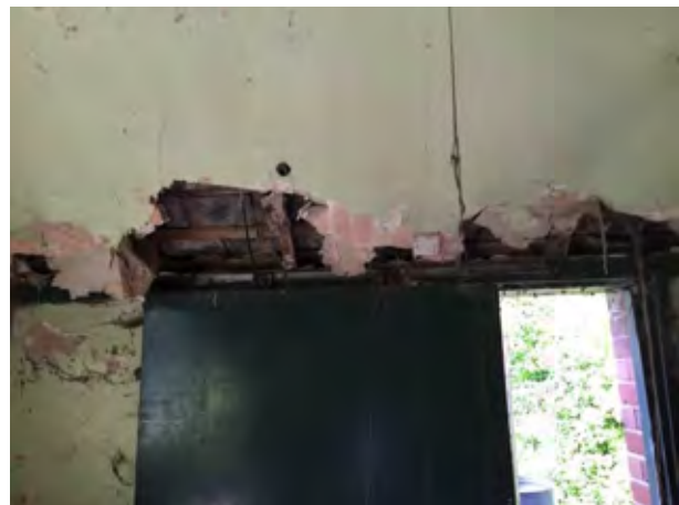
Holes through roof at eaves level on front elevation, Room 1.
