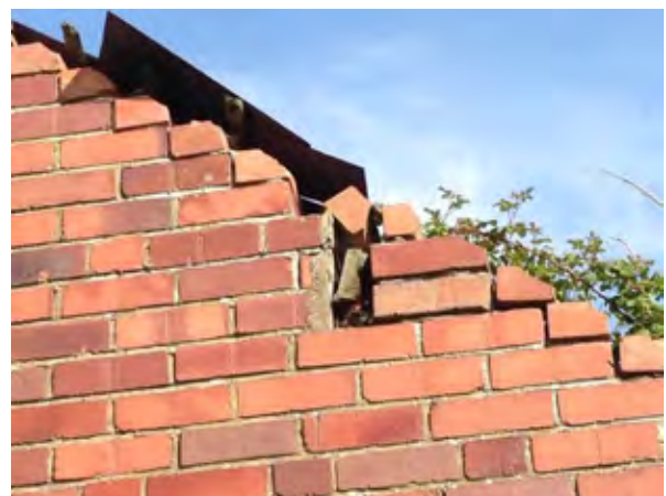
Damage to brickwork and rotten roof timbers visible. Verge mortar missing.
