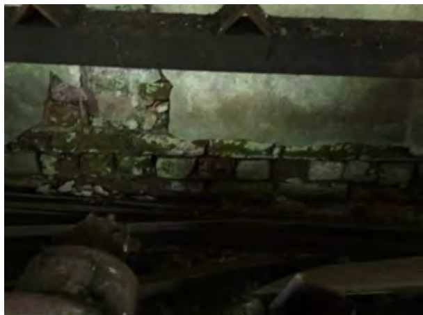
Water staining to rear wall, Room 4.
