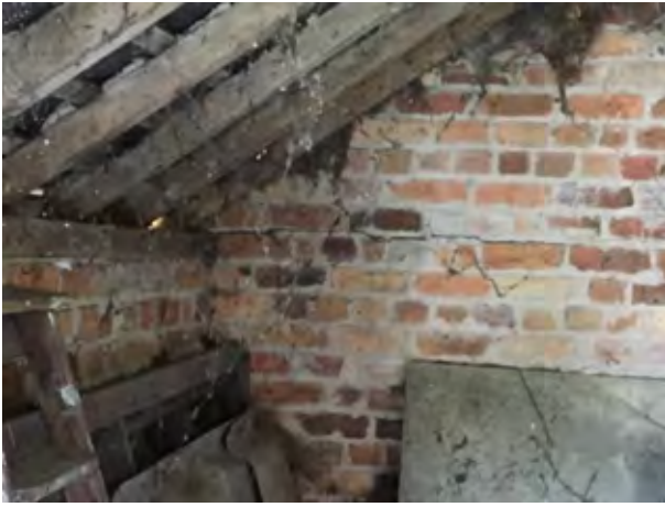
Horizontal cracking at eaves level.
