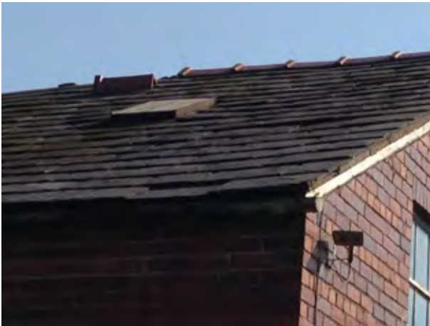
Slipped slates and ridge tiles.
