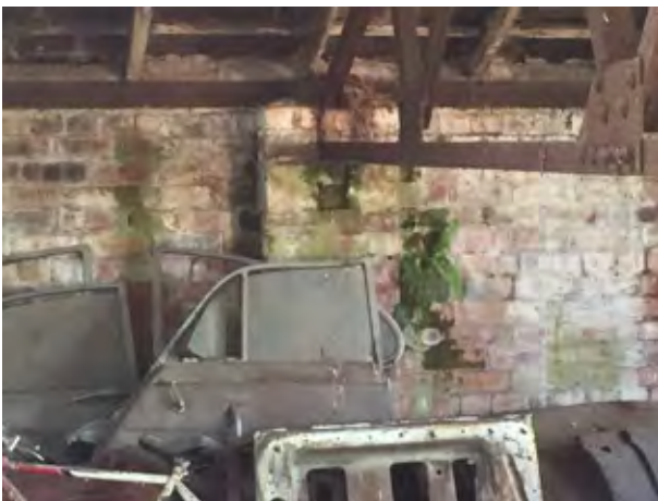
Water staining to left hand side wall.
