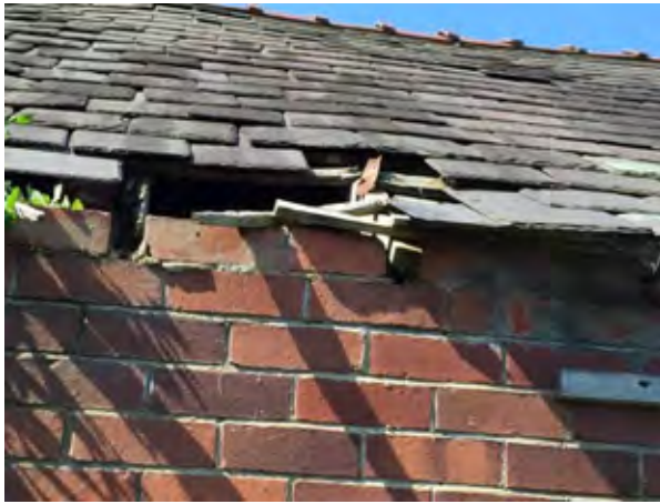
Holes through the roof at eaves level. Rafter ends rotting.
