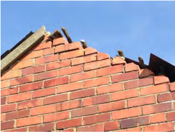
Edge of roof damaged.
