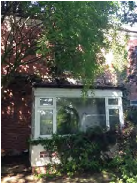
Porch structure partially covered by vegetation.
