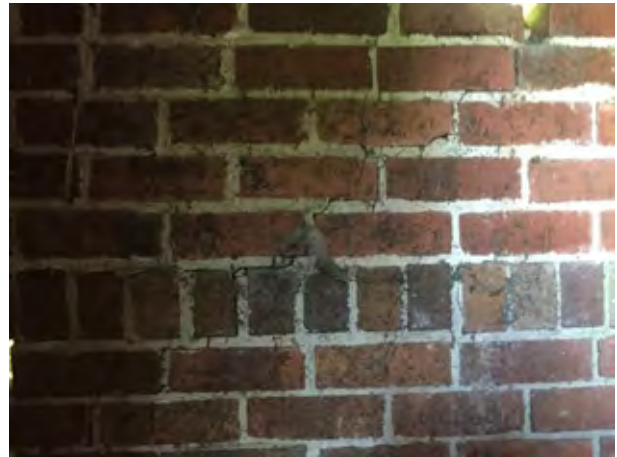
Cracking continues onto front wall.
