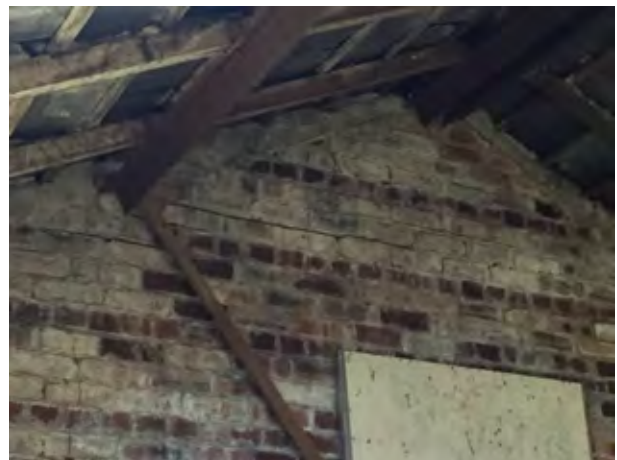
Cracking and brickwork lifting on front elevation, internally.
