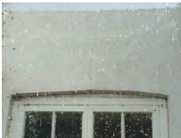
Cracking to brick arch lintel to side elevation within the rear porch structure.
