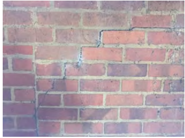
Stepped cracking to right hand side gable wall.
