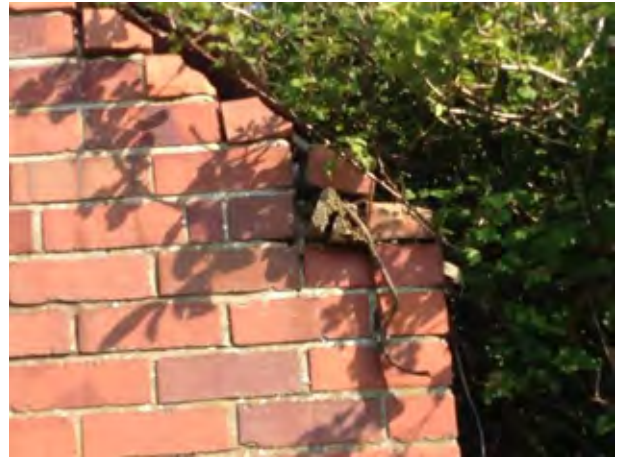
Wall plate rotting. Slate over hang missing.
