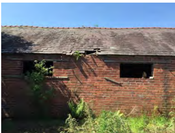
Undulating roof. Holes through roof at eaves level.
