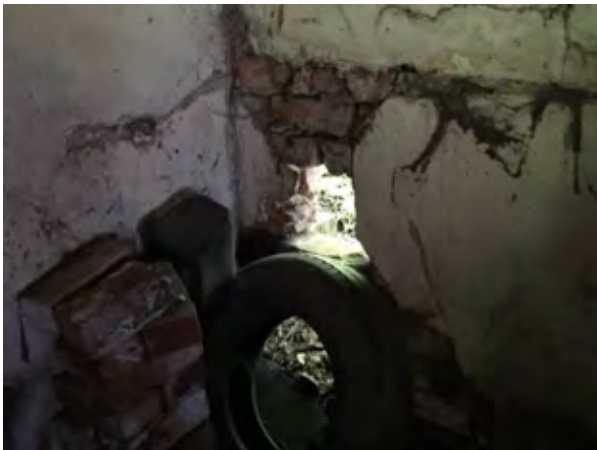
Hole through wall in Room 4.
