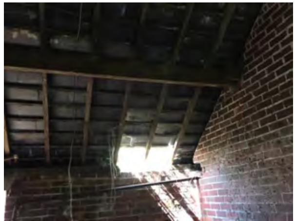
Holes through the roof.
