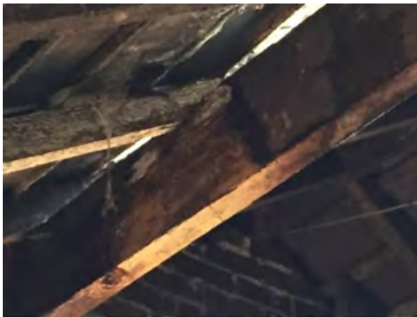
Water staining to timbers.
