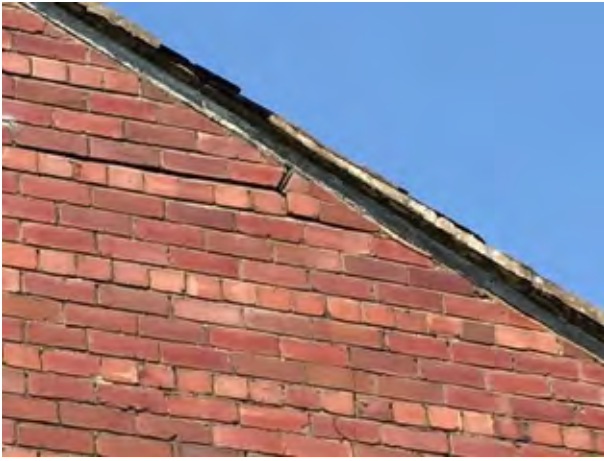
Cracking and lifting brickwork where purlin end built into elevation.
