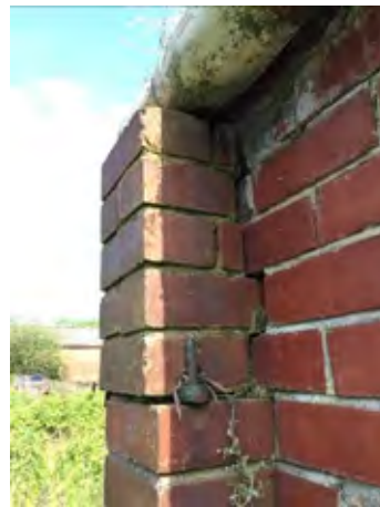
Cracking and movement of pier / buttress.
