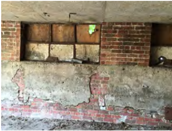
Steel window frames supporting elevations. Render dislodging.
