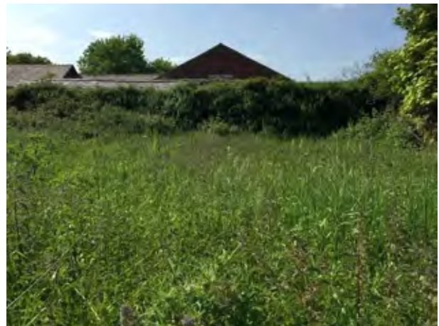
Vegetation growing up the face of the structure.
