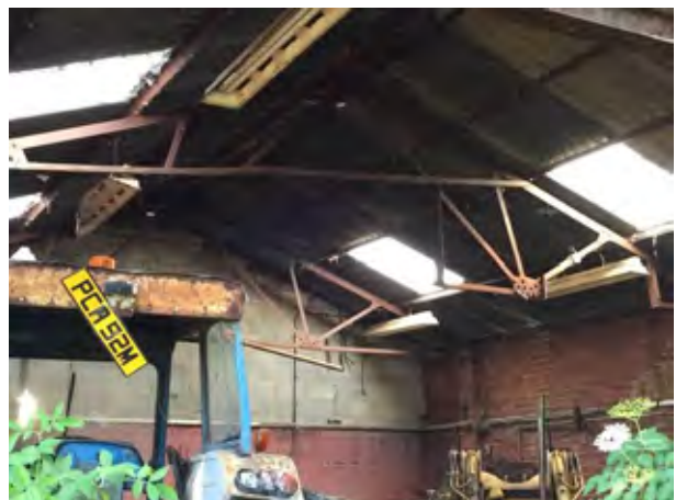
Trusses with bottom chords missing.
