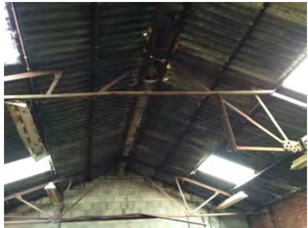
Bottom chord missing from steel truss.
