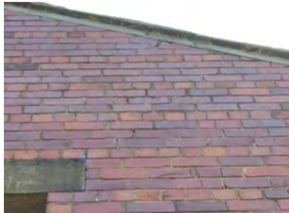
Cracking to the right hand side of the central opening at first floor level.
