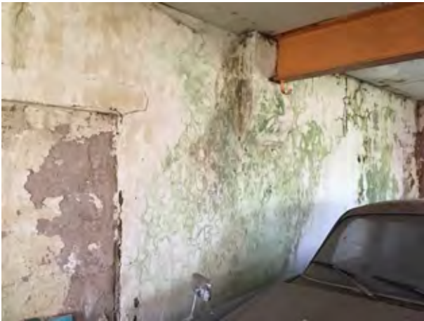
Staining to left hand side wall.
