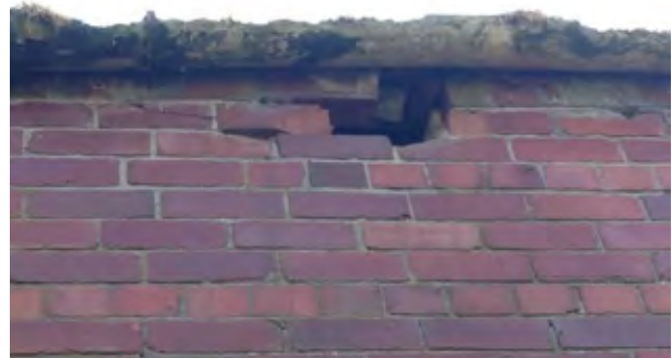
Holes through elevation and damaged gutters which may contain asbestos.
