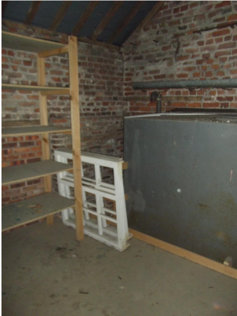
Picture 16 Internal storage tank at first floor level
