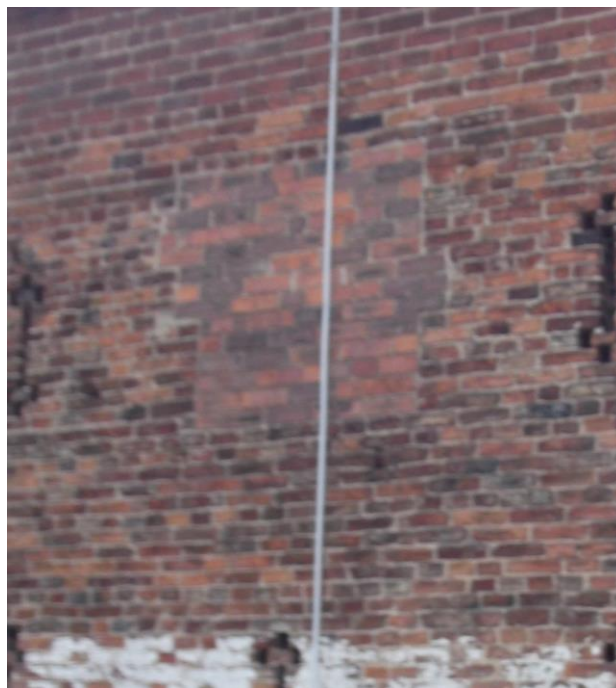
Picture 6 Blocked up opening which is to be reopened
