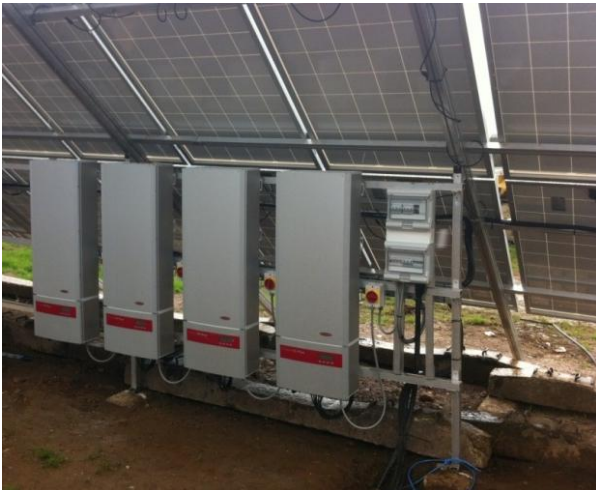
"String" Inverters mounted on frame structure below the panels
