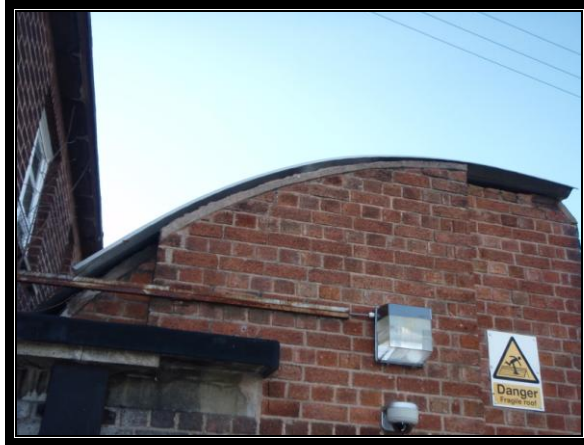
Potential gaps at Target Note 13a (where corrugated roof separates from brick walls).
