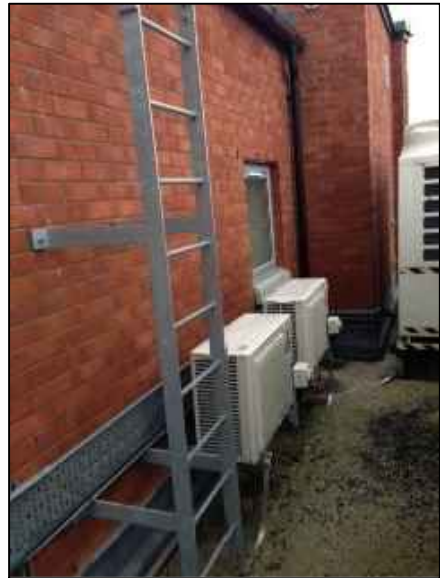
EXISTING OUTDOOR UNITS
