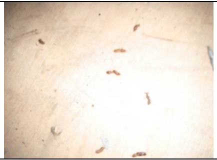
Scattered brown long-eared bat droppings commensurate with single/small numbers of bats, found within loft space of residential accommodation.
