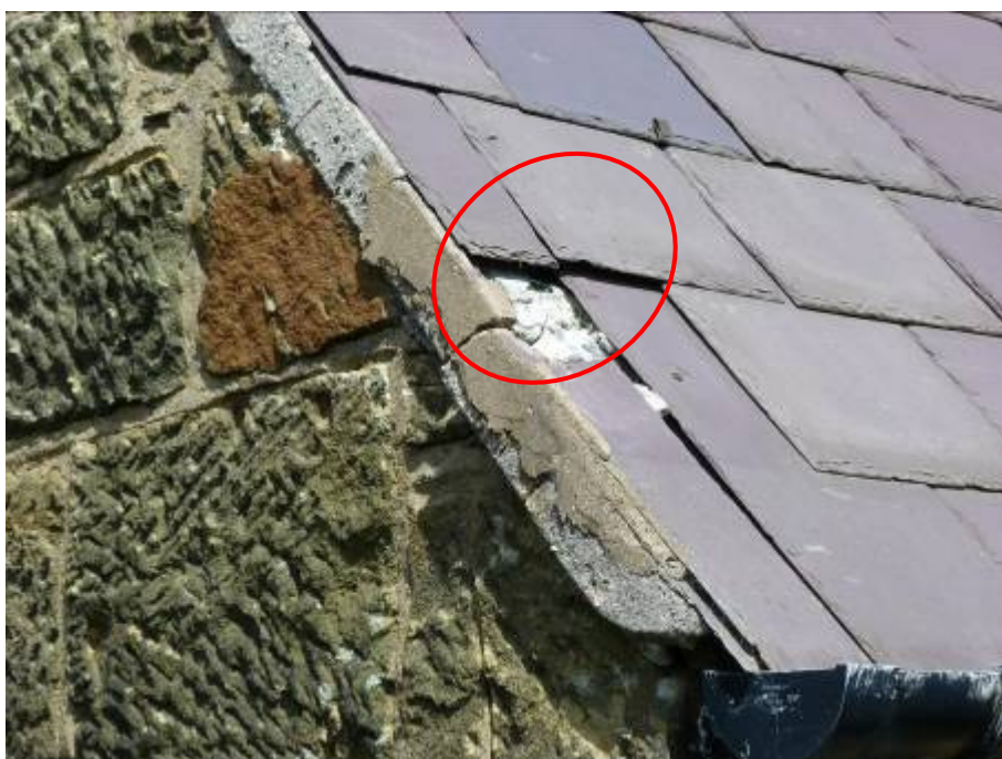
Gaps in extension roof void, slipped slates & roof verge on main building
