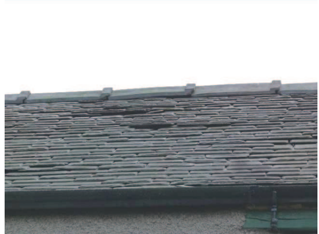
Photo 6: Showing slipped/raised/missing roof slates creating potential bat access points.
