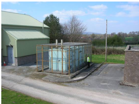
Photograph 4: View of compound housing backup generator within wire enclosure and shallow concrete bund. Electricity sub station / transformer house is located to right of photograph. Chemical house is located to the left of the photograph.
