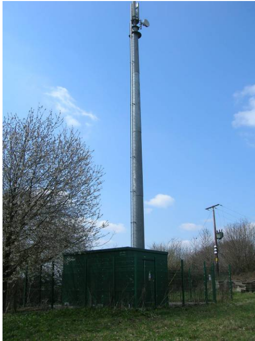
Photograph 13: View of telephone mast located at the western boundary of site.
