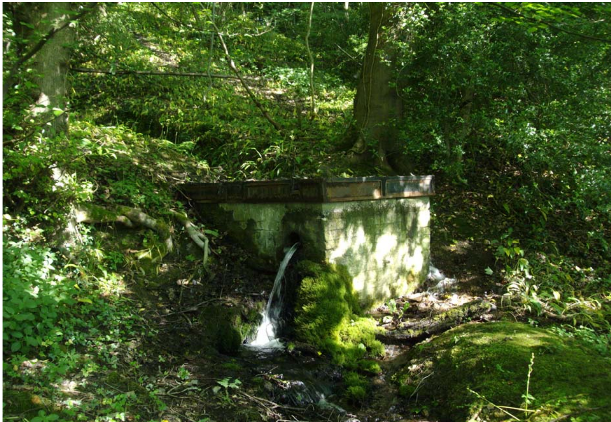
Photograph 12: Block enclosure and discharge
