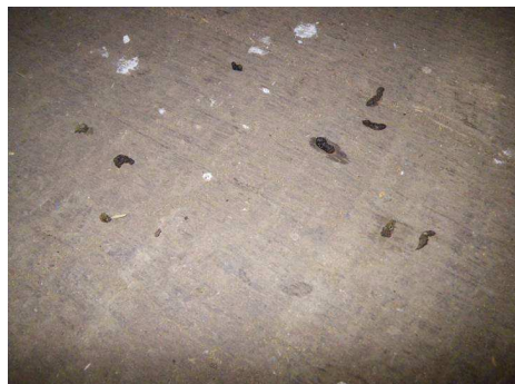
Figure 8 - example of bat droppings found on first floor
