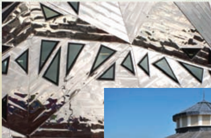
The Public, West Bromwich Alsop Architects Bespoke Triangular Rooflights
