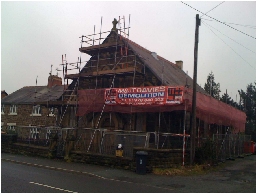
Picture 2 Extent of disrepair to front and side elevation
