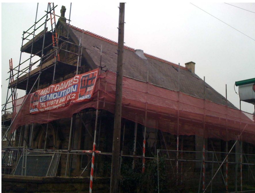
Picture 3 Extent of wall and roof disrepair from side elevation
