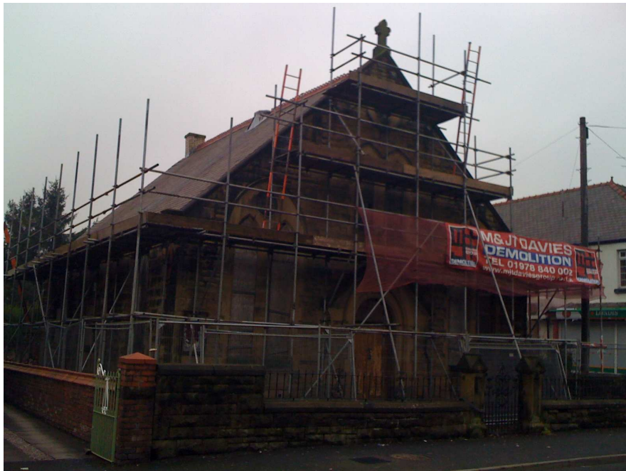
Picture 1 Extent of disrepair to front and side elevation
