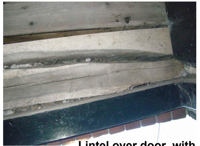
Lintel over door, with crevices
