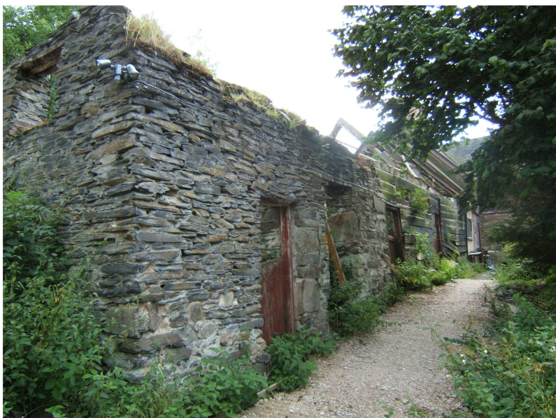
View of front – the derelict part at LH side (north) of farmhouse
