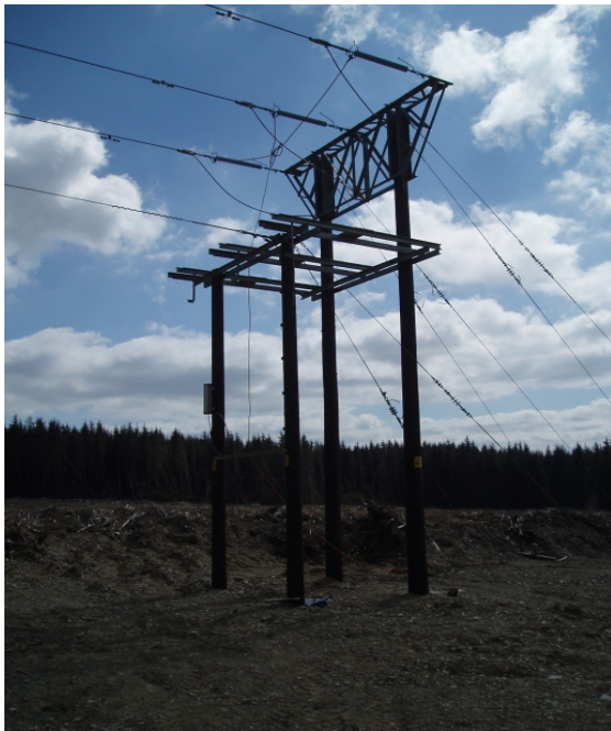
7. Terminal (4 pole) structure; with stays
