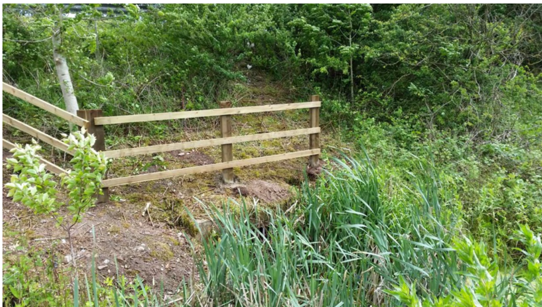
Images 3.2: Facing east: Shows overgrown headwall as water is culverted under elevated A483
