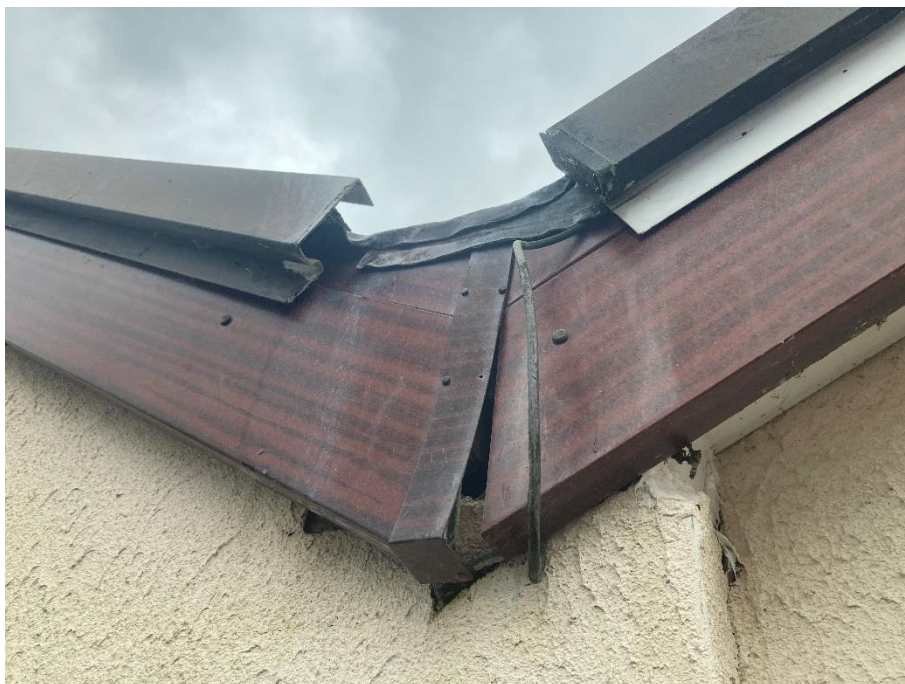
A1.7 Plate 7: Gap beneath cap of barge board on western aspect (front) and access under roof tiles.
