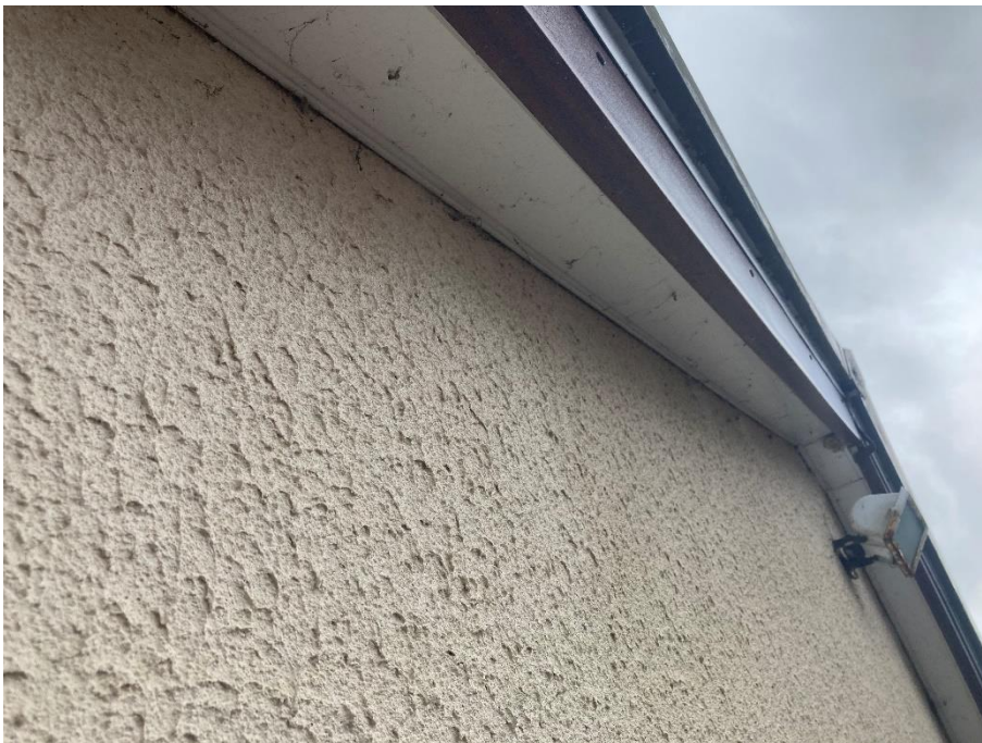
A1.4 Plate 4: gable end barge boards well sealed no gaps for bats
