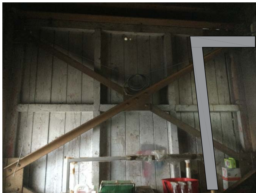
PHOTO 05 - PHOTO MONTAGE OF CABLE TRAY WITHIN STORE TO SUPPLY TELECOMS CABINET ON PLATFORM 2/3
