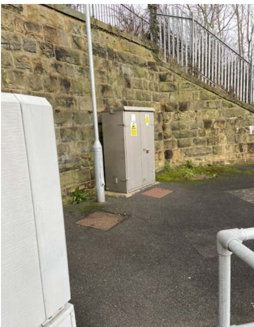
PHOTO 05 - EXISTING FEEDER PILLAR CONTAINING DISTRIBUTION BOARD DB6 LOCATED ON PLATFORM 1 TO SUPPLY NEW CIS SCREEN
