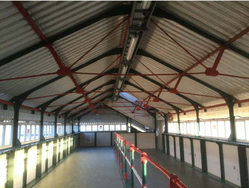
PHOTO 02 - EXISTING CABLE TRAY OVER BRIDGE, USED TO FEED NEW DISTRIBUTION BOARD TEL/1 ON PLATFORM 2/3
