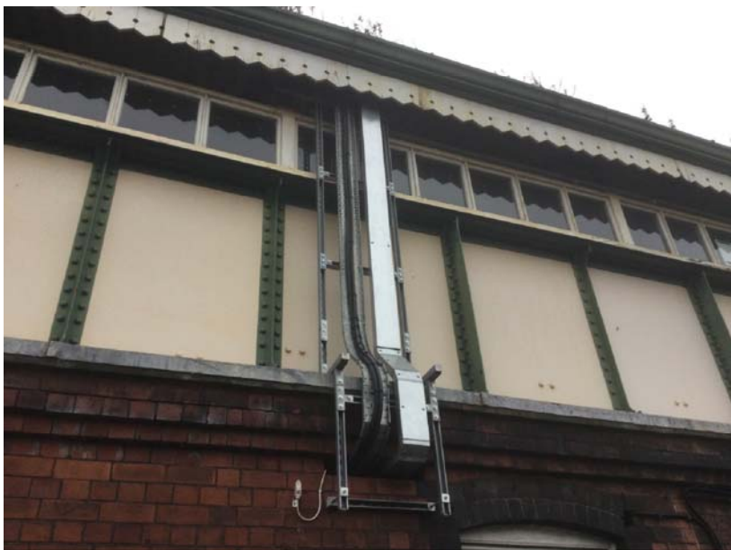
PHOTO 01 - DBA/1 - EXISTING CABLE TRAY RUN FROM STORE AND OVER BRIDGE, USED TO FEED NEW DISTRIBUTION BOARD TEL/1 ON PLATFORM 2/3
