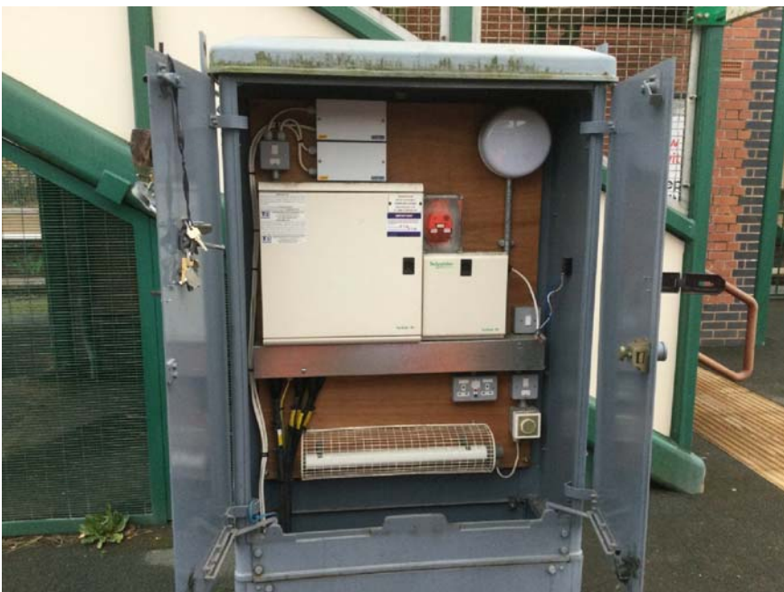
PHOTO 04 - EXISTING CABINET ON PLATFORM 4 SHALL SUPPLY NEW TELECOMS CABINET DISTRIBUTION BOARD TEL/2 ON PLATFORM 4
