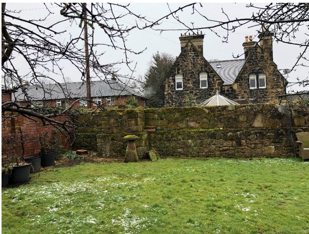
FIG5 – view back toward house of central wall, heavily rebuilt in recent years
