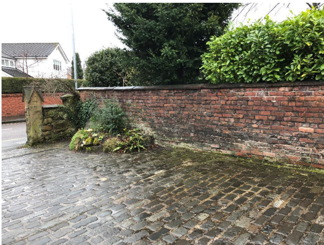
FIG8 – view of SW boundary wall to driveway, with heavy inward lean
