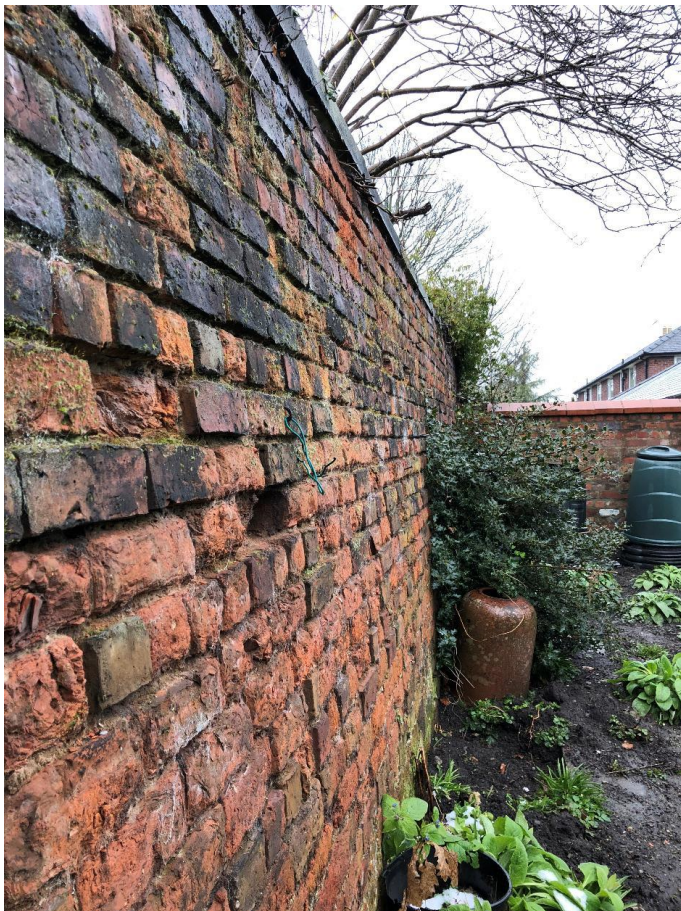
FIG4 – photo showing dramatic lean toward neighbouring side, note later bricks at high level
