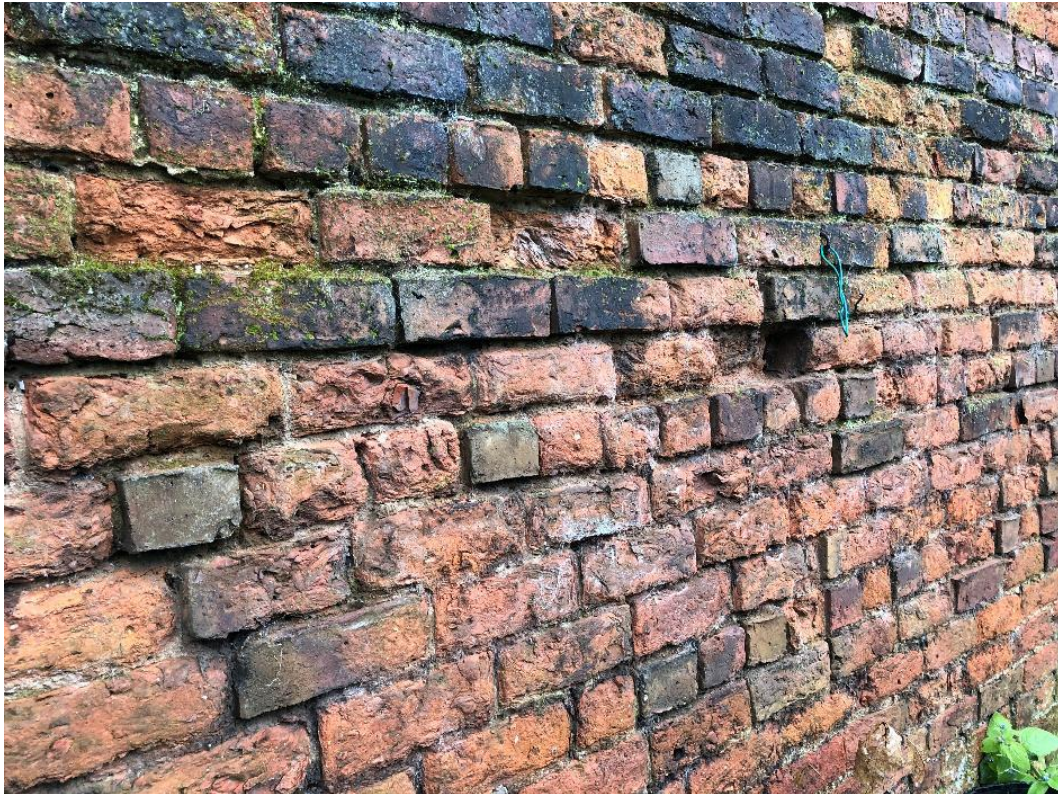
FIG3 – Close up photo of the wall showing poor condition of brickwork
