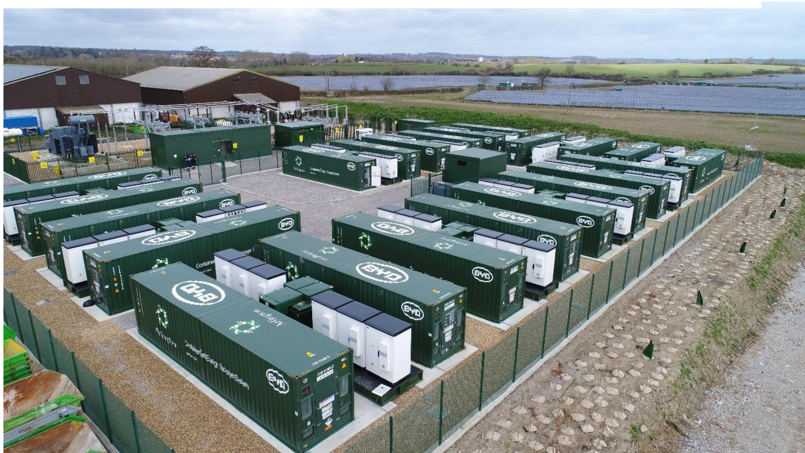
Figure 8: Example of a battery storage facility
