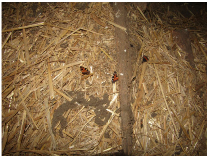
Photo 6: Scattered butterfly wings were observed in the upper level near the East gable-end.
