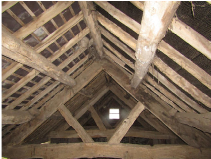
Photo 4: Felt beneath slates only on South pitch of roof.
