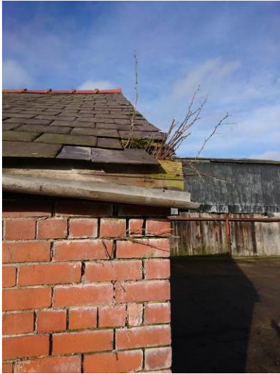
Photo 6 – Vegetation growing from wall plate.
