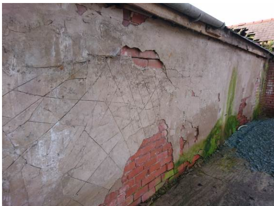
Photo 14 – Inwards bulge in wall.
