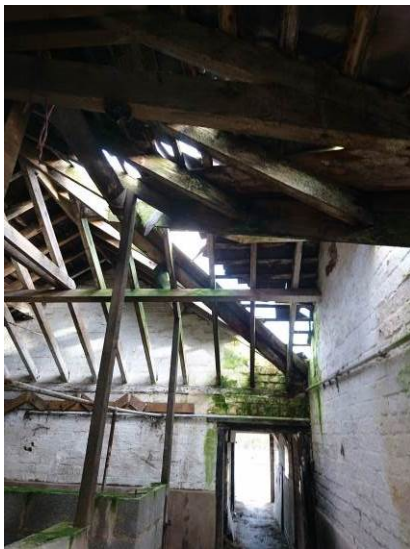
Photo 19 – Missing slates to roof.
