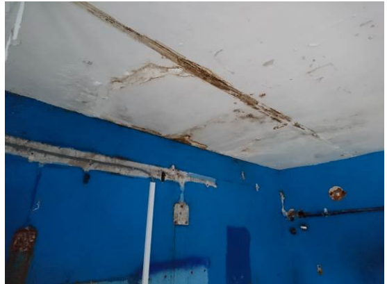
Photo 26 – Staining to ceiling finishes.
