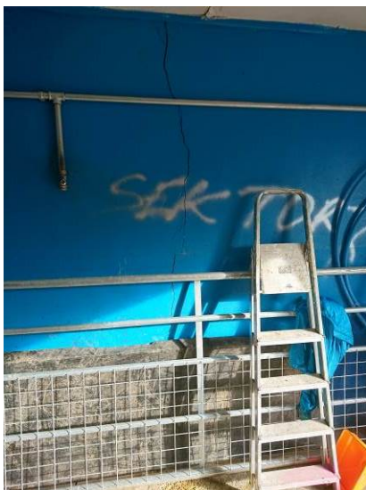
Photo 25 – Cracking to internal wall.
