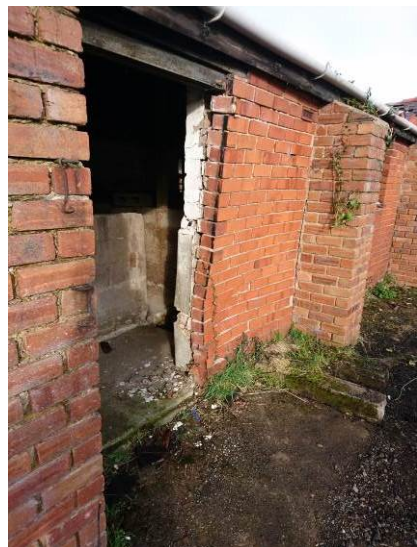
Photo 5 – Impact damage to elevation.
