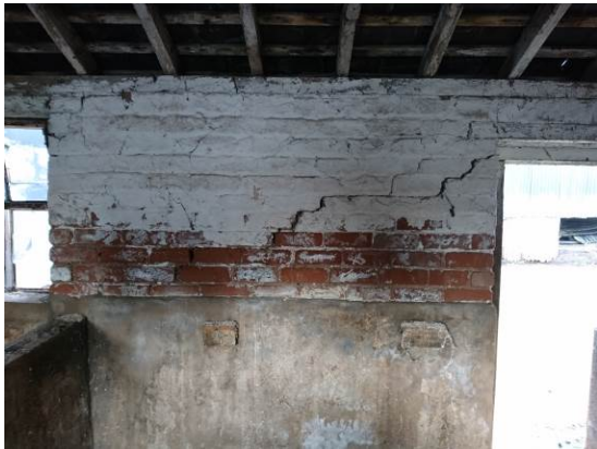
Photo 18 – Cracking to rear elevation.
