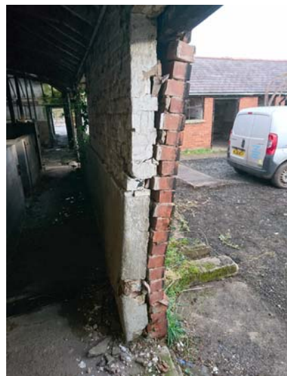
Photo 17 – Impact damage to brickwork.
