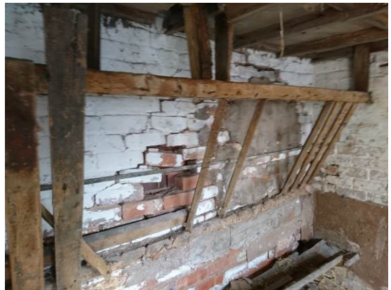
Photo 21 – Severe inwards bulge to wall.
