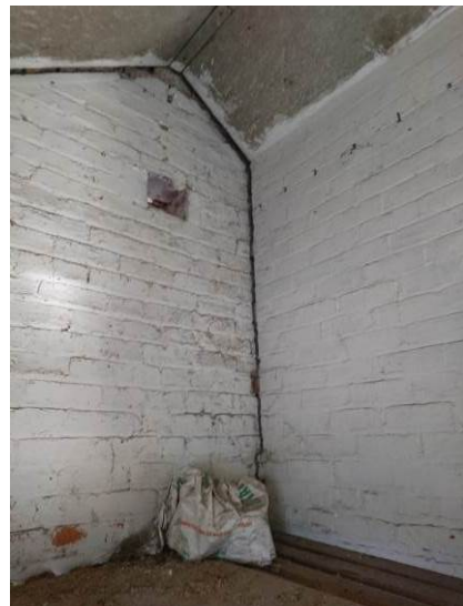
Photo 23 – Gap between internal and external walls.
