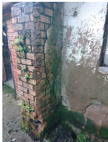
Photo 11 – Severe erosion to buttress.
