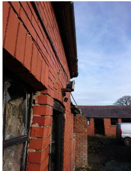
Photo 4 – Dislodged arch over opening and brickwork above.
