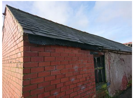
Photo 15 – Fire damage to fascia and lintel.
