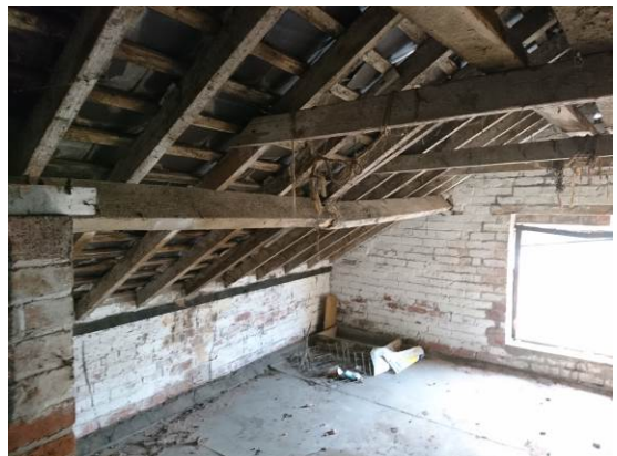
Photo 27 – Broken purlin and additional ceiling ties.
