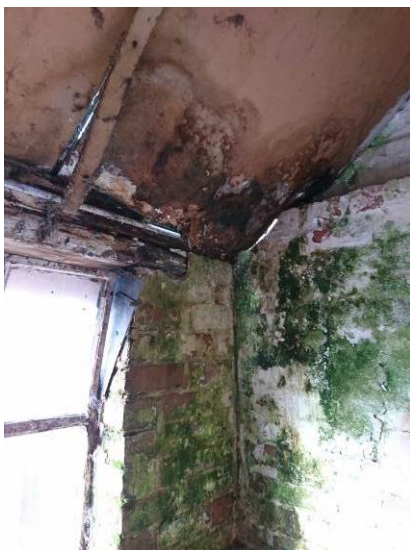
Photo 20 – Weather penetration below valley.
