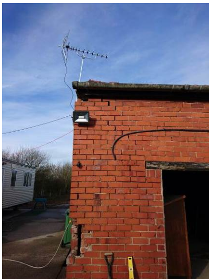
Photo 3 – Cracking above door opening.
