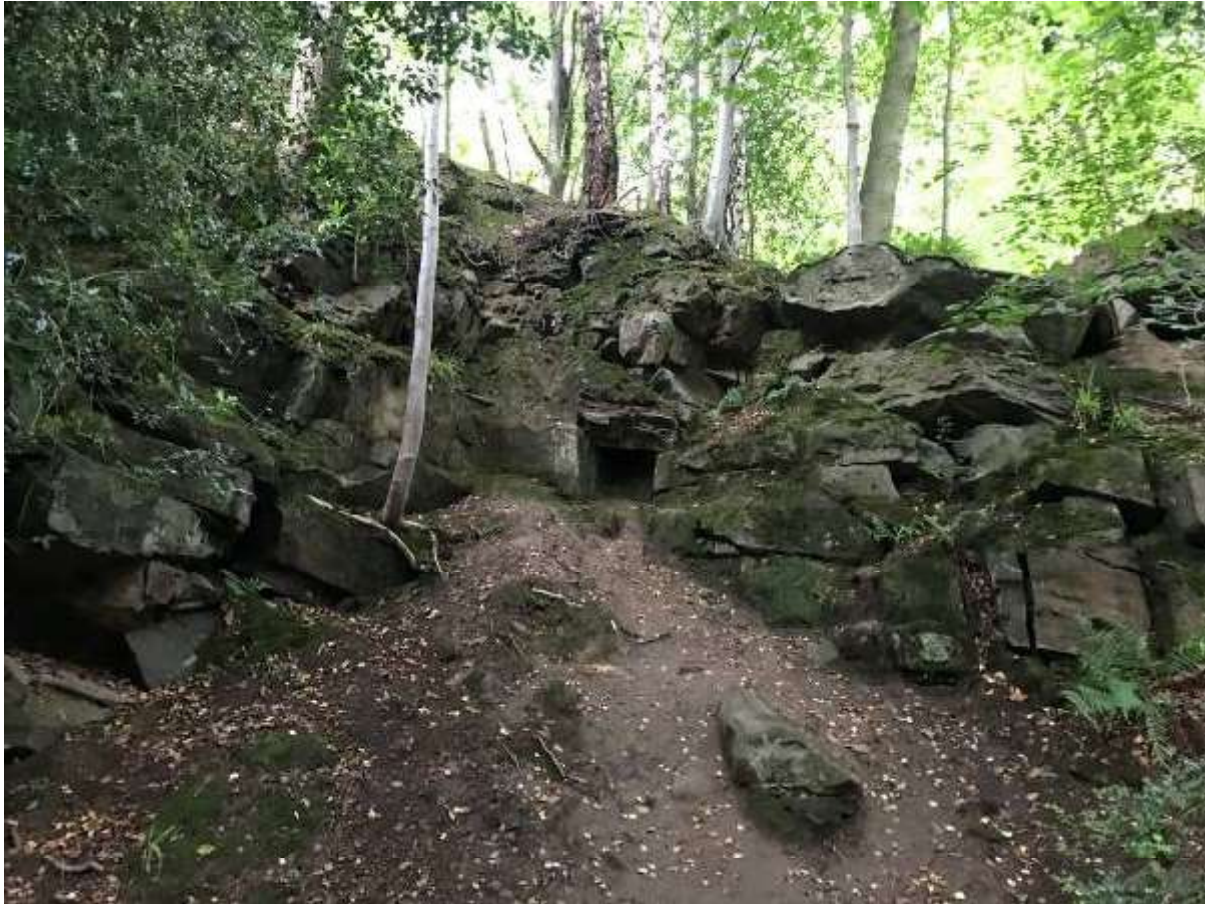
Photo 5 – displaced clocks and rock face along path (up to 25m from gate)
