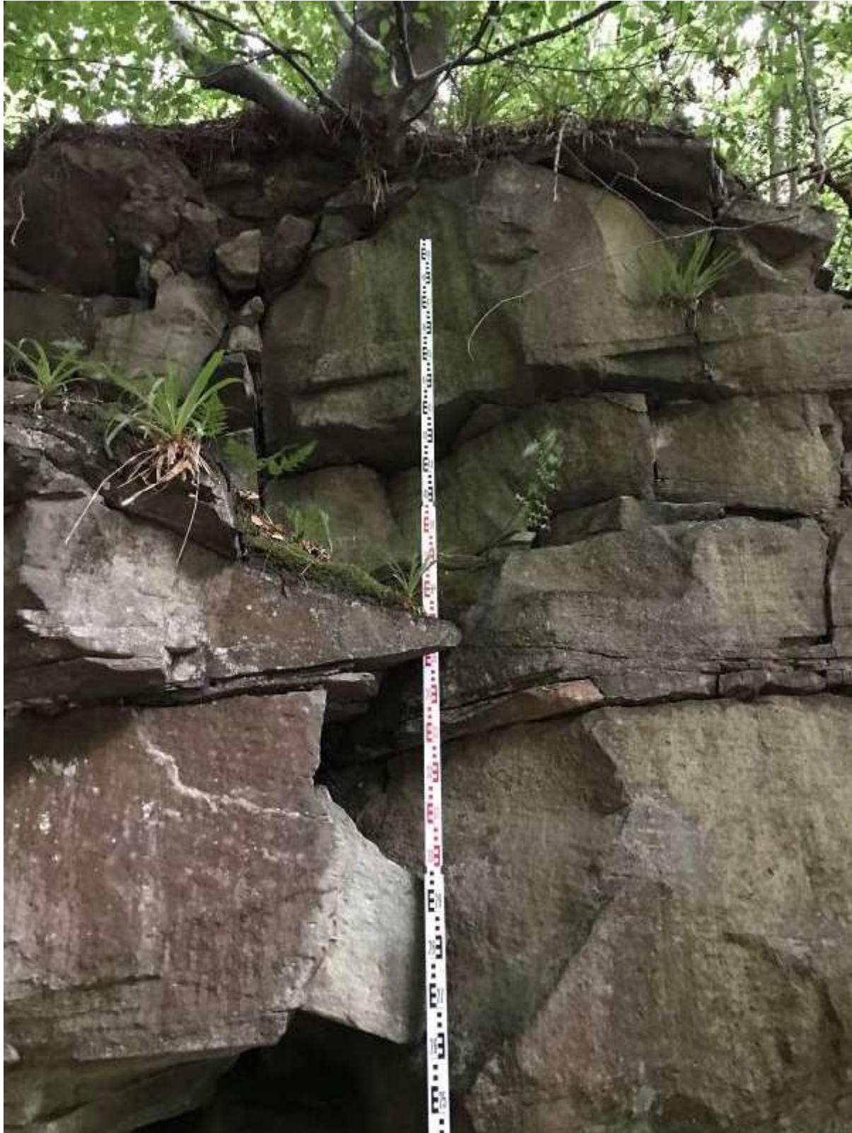
Photo 3 Area 1 – dilated joints and root penetration
