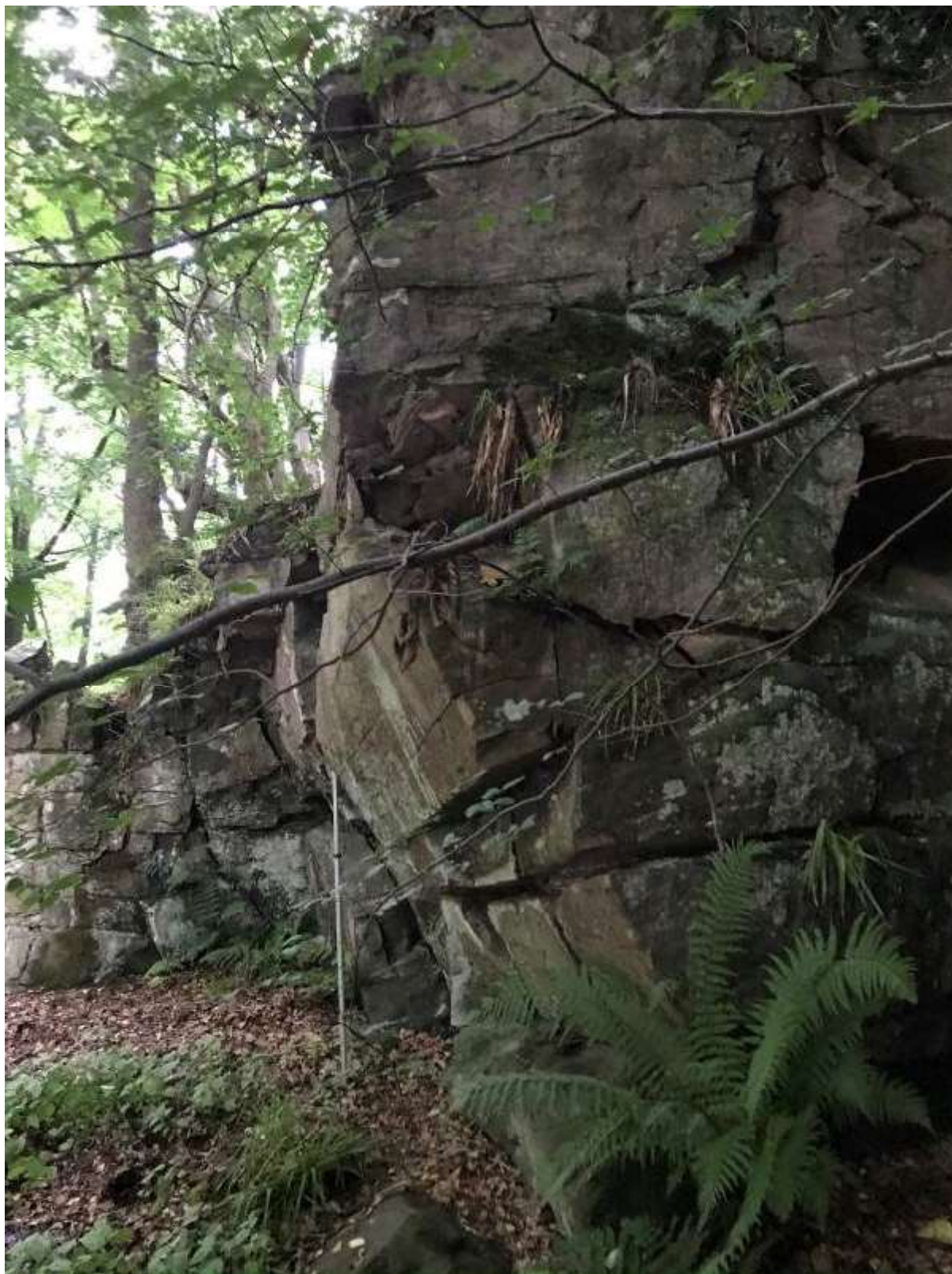
Photo 2 – 6m section closest to listed wall – unfavourable dip of fractures
