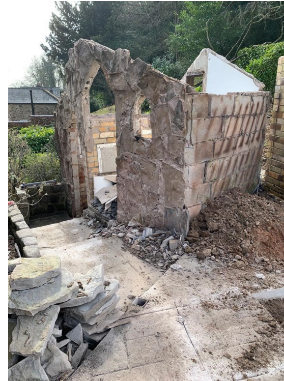
Image 1- Front of Plant Room
