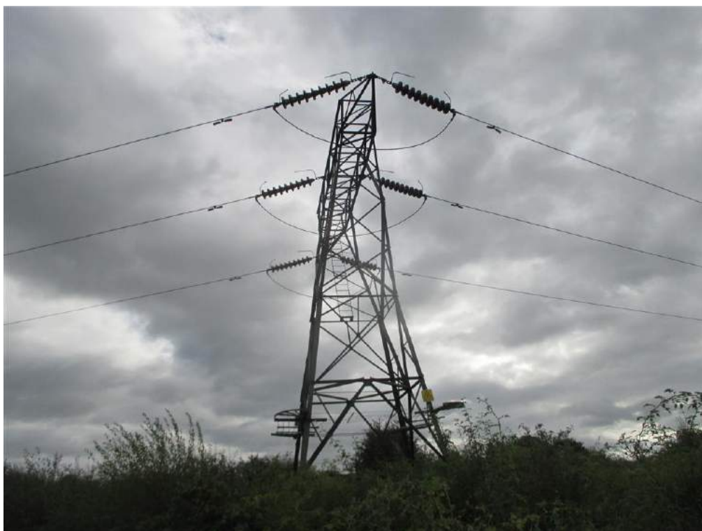
Plate 7: Typical metal lattice electricity pylon.
