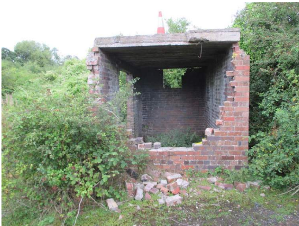
Plate 10: Example of a damaged building in the north east area of the site.
