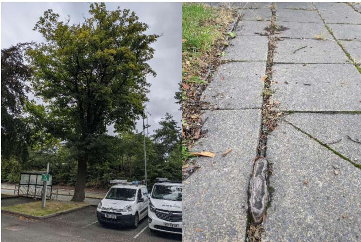
Figure 46. Tree 34 (sycamore) Crown size and structure (left). Roots pushing up between flags (right).
