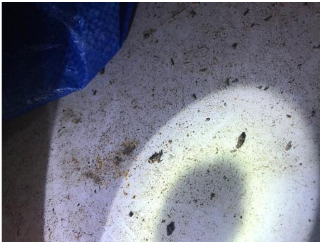
Plate 13 – Droppings attributed to Pipistrellus sp. bats, located in the western wing
