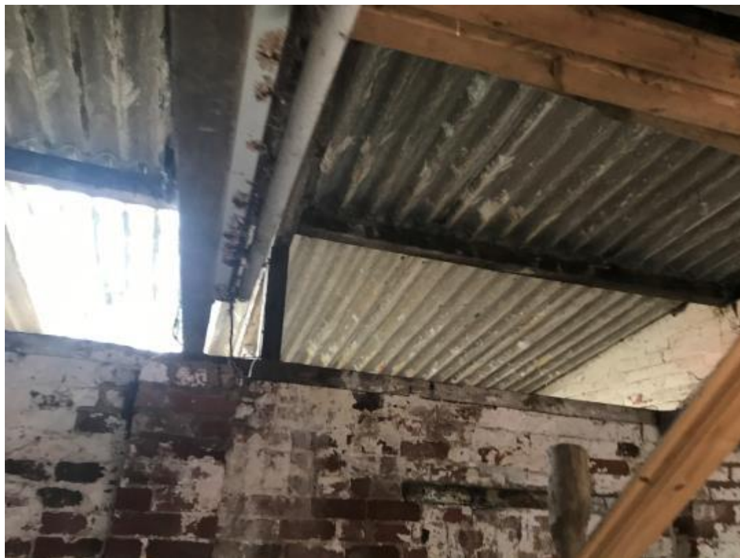
Plate 11 – Open ingress point via the lean to on the north-western wing
