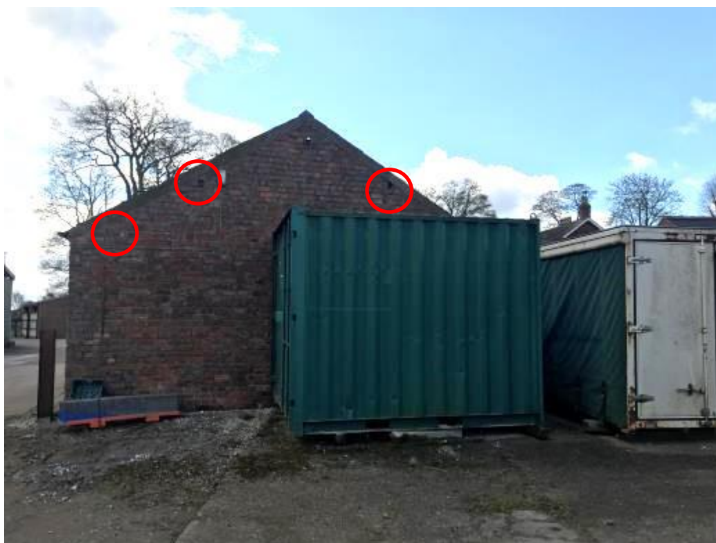
Plate 6 – Northern elevation of the eastern wing with gaps in the brickwork
