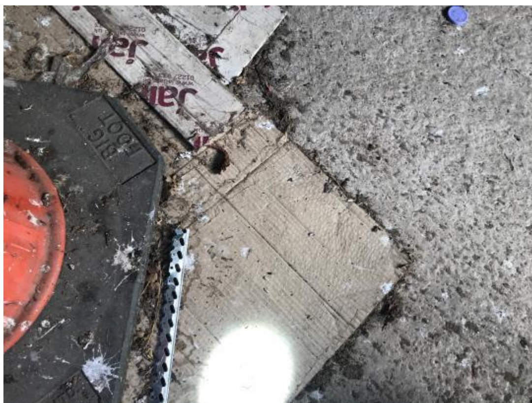
Plate 12 – Bird droppings within the barn
