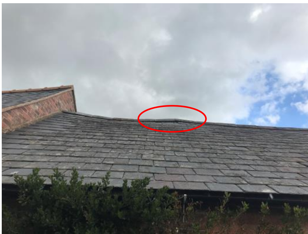
Plate 2 – Gap beneath ridge tiles on the western wing
