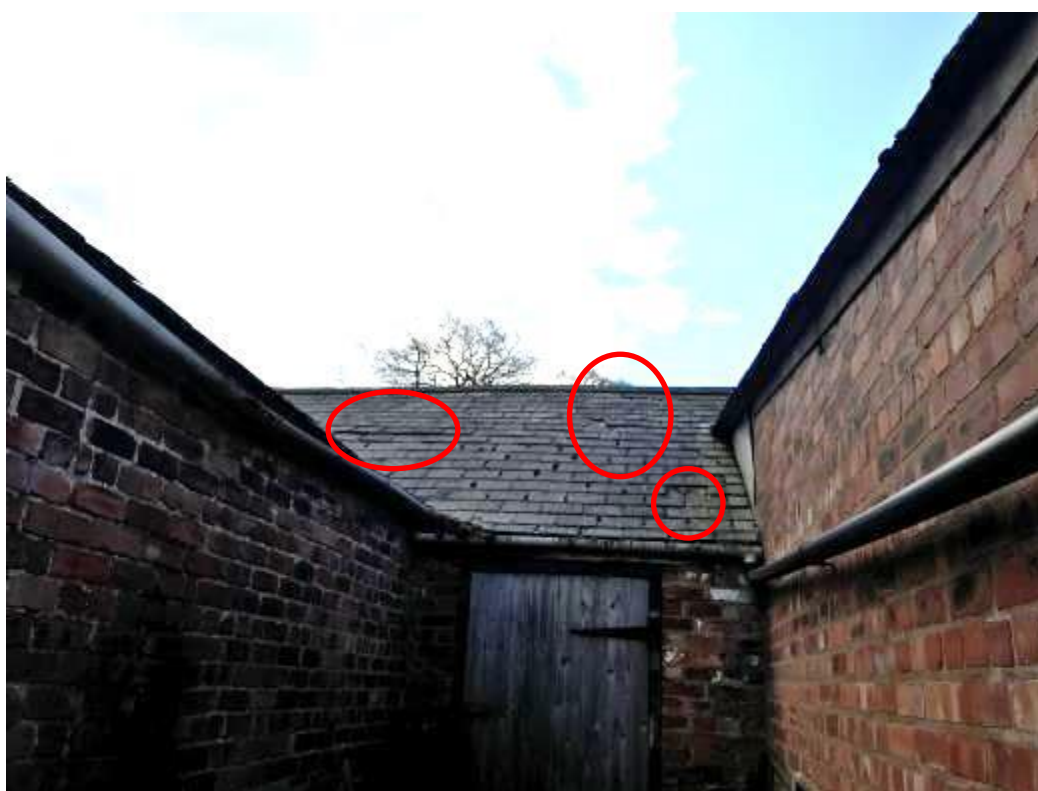
Plate 8 – Area between eastern and western wings, with gaps beneath slates
