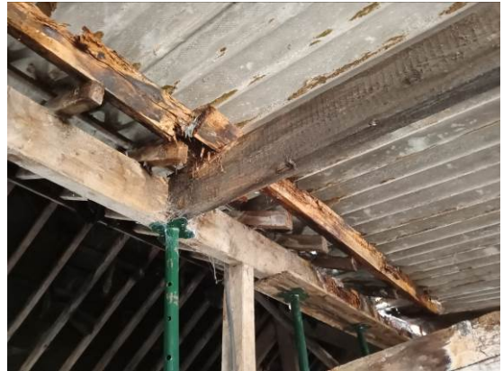
Photo 15 – Severe rot to timbers. Note propping to timber beam.
