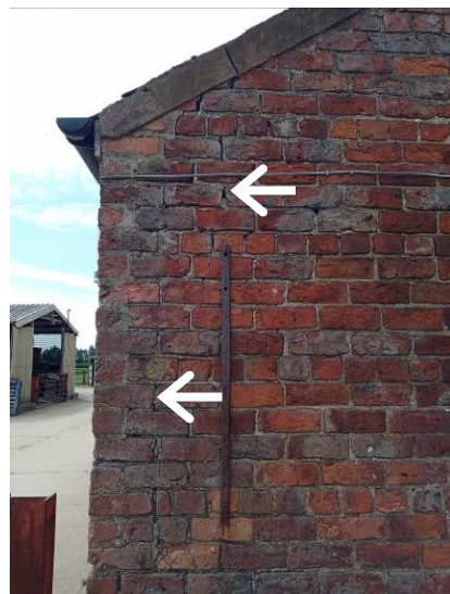
Photo 6 – Cracking extending down from eaves.
