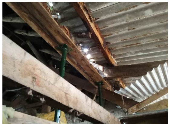
Photo 16 – Severe rot to timber with props to underside.
