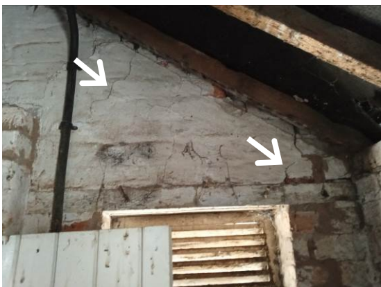
Photos 9 – Cracking above opening.
