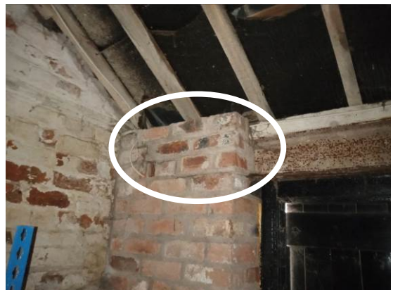
Photo 12 – Dislodged brickwork at lintel end.
