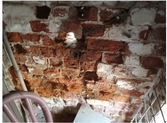
Photo 10 – Erosion to brick units.
