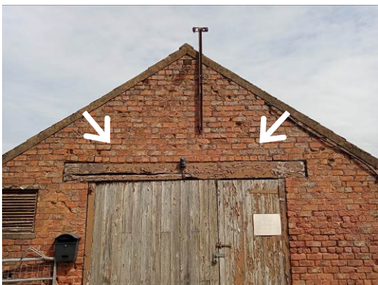
Photo 3 – Cracking extending from timber lintel. Note: sag to bed joints over lintel.
